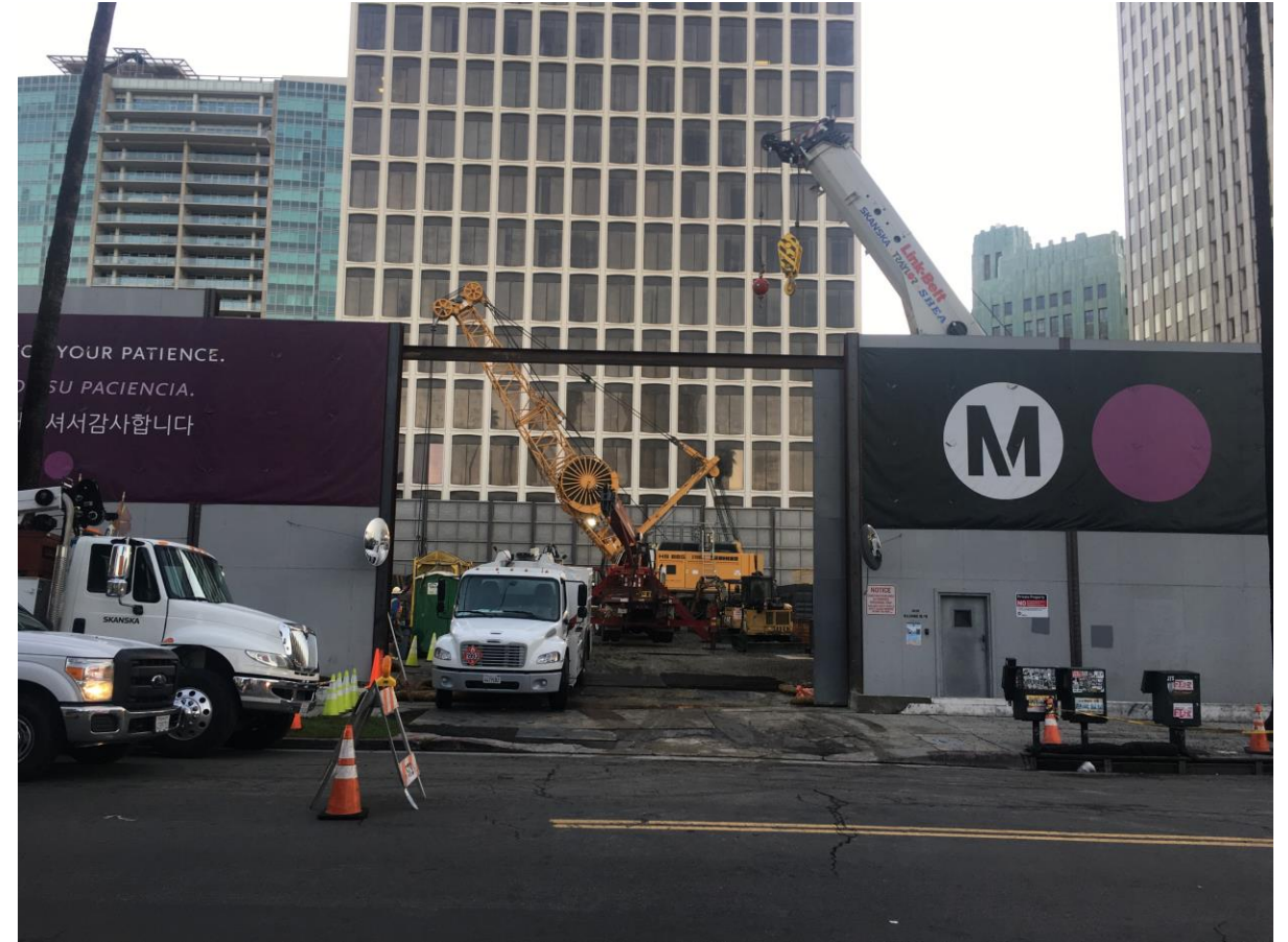
Relief Shaft – Wilshire/Western
