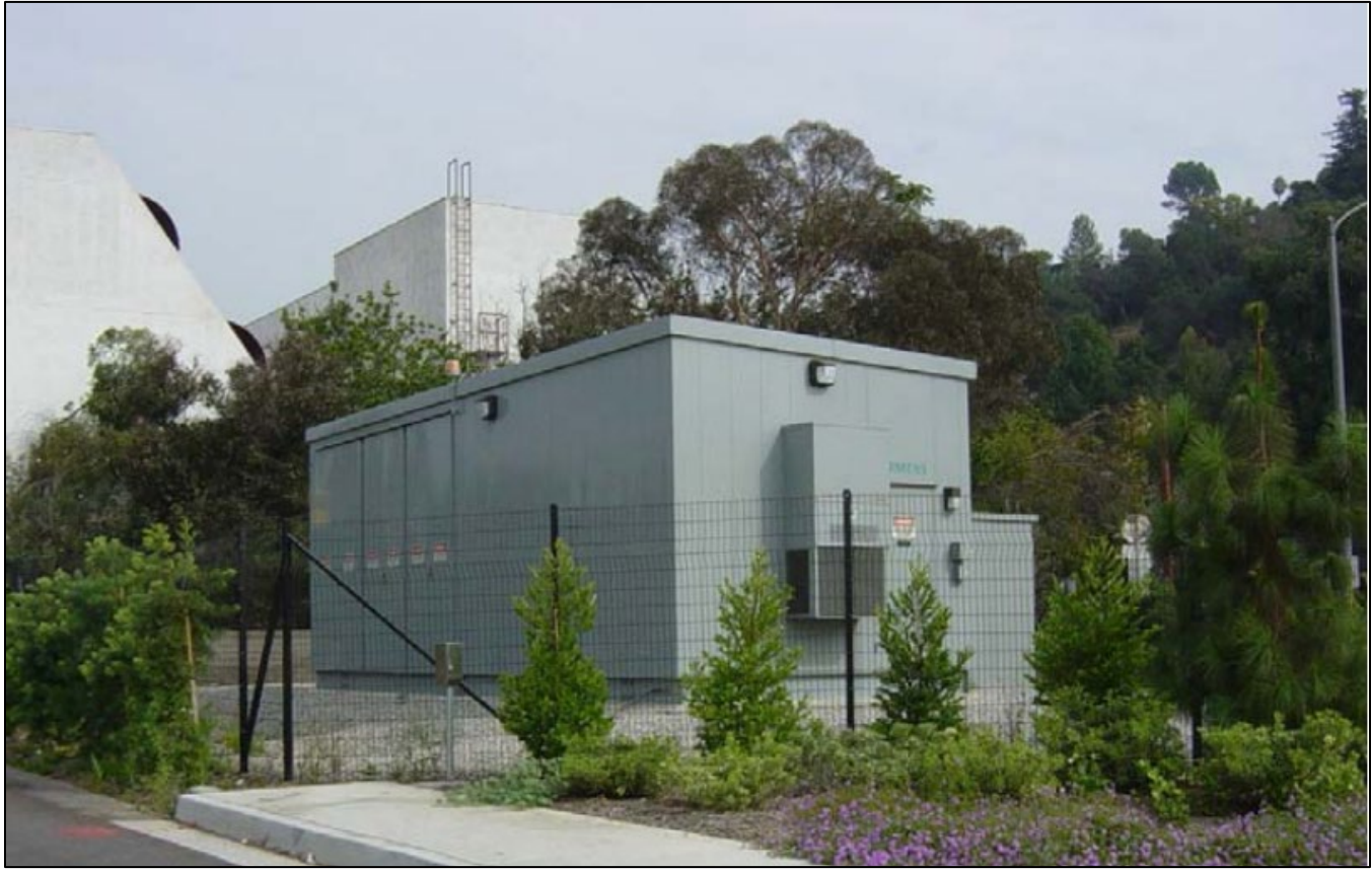
Source: Metro Gold Line Foothill Extension Construction Authority 2012. Figure 2.10 Typical Light-Rail Traction Power Substations
