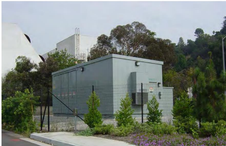
Figure 2.4-3. Typical TPSS Facility
