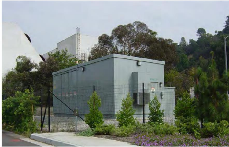
Figure 2.3-33. Typical TPSS Facility
