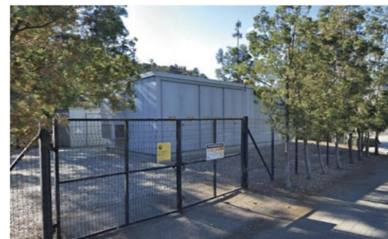
Traction Power Substation
