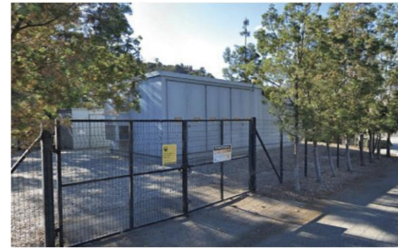
Traction Power Substation
