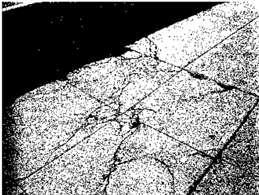
Perimeter sidewalks require repair.
