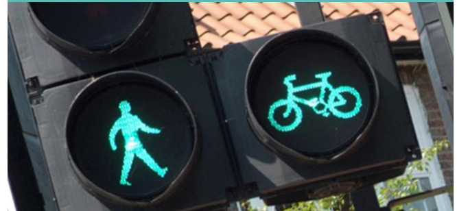
Bike/Pedestrian Traffic Controls
