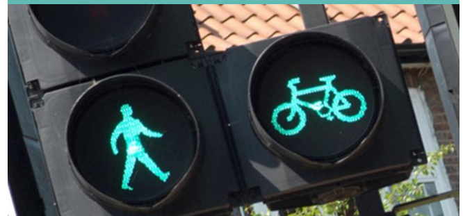
Bike/Pedestrian Traffic Controls
