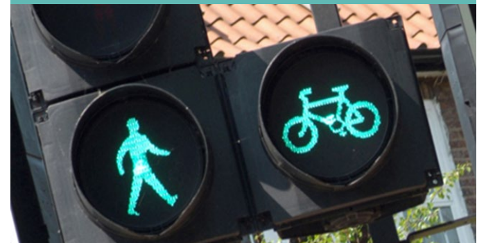
Bike/Pedestrian Traffic Controls
