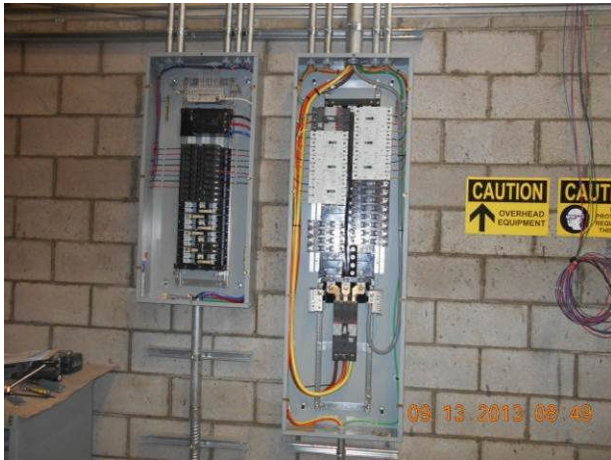
Control panel for electrical system at Radiator Shop.
