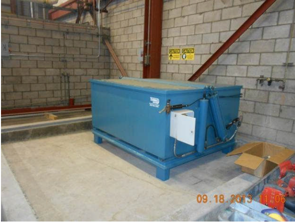
Boil out tank equipment at New Radiator Shop.
