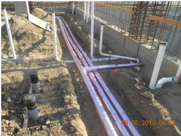
Domestic water and sewer pipes at Transportation Bldg.
