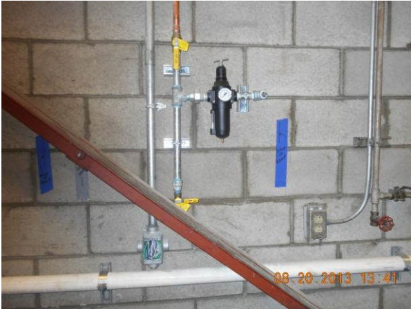
Compressed air equipment at new Radiator Shop.
