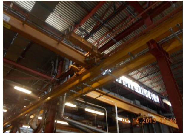
Electrical conduit attached to ceiling structure at Radiator.
