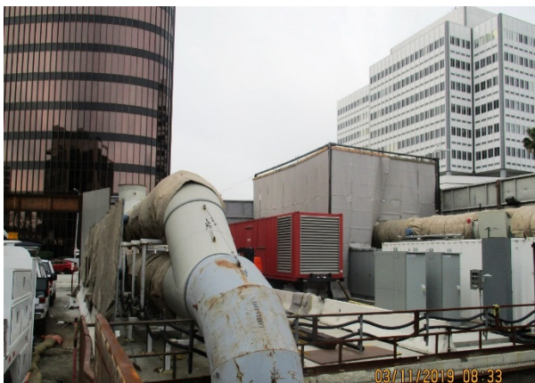
Ventilation System at Wilshire/La Cienega Station
