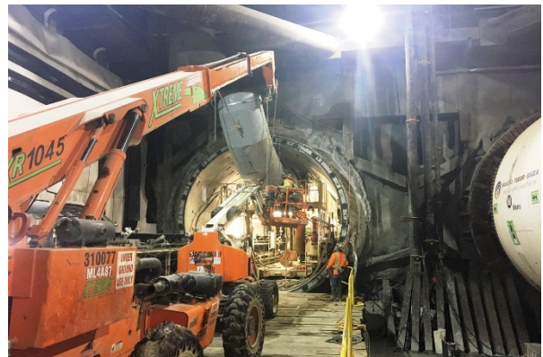
Wilshire/La Brea Station – Hanging Ventilation
