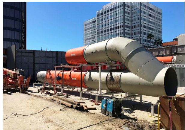
Ventilation Ducts at Wilshire/La Cienega Station
