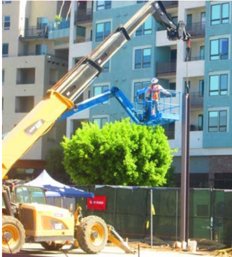
C1045 Contractor Installing Columns for the Soundwall at the South Wilshire/La Brea Construction Staging Site
