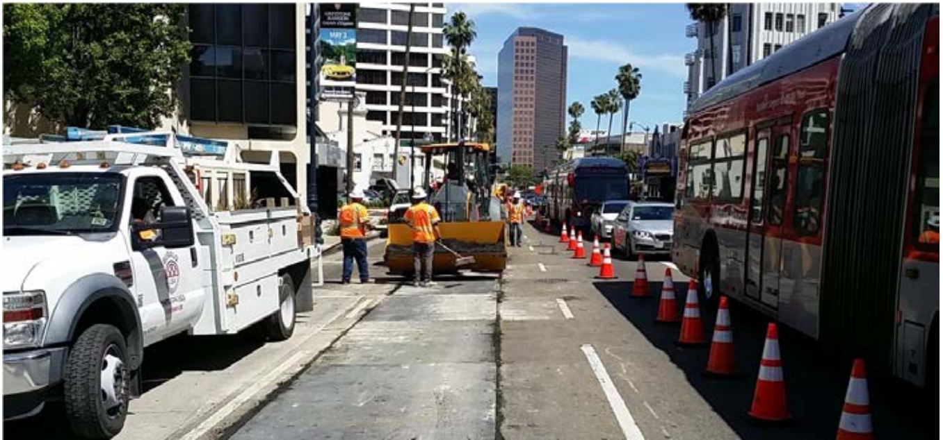
C1056 Wilshire/La Cienega AUR Contractor Placing Steel Trench Plates above Utility Trench
