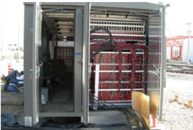
Operations Campus: Train Control Bulgalow Wiring
