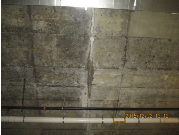
Water leaks in parking garage.
