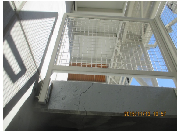
Concrete slab crack appearance at Parking Garage Level 1.
