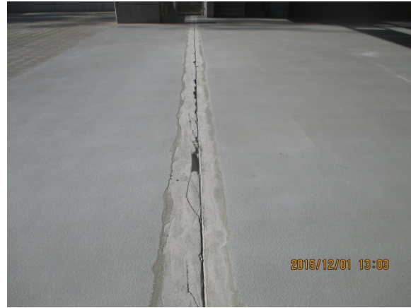
Cracks in concrete slab in parking garage.
