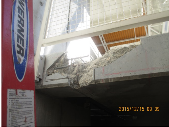
Broken concrete slab crack to repair.
