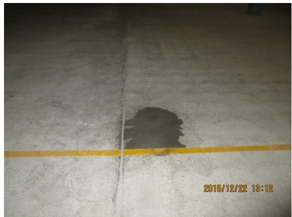
Water leaks in parking garage from roof.
