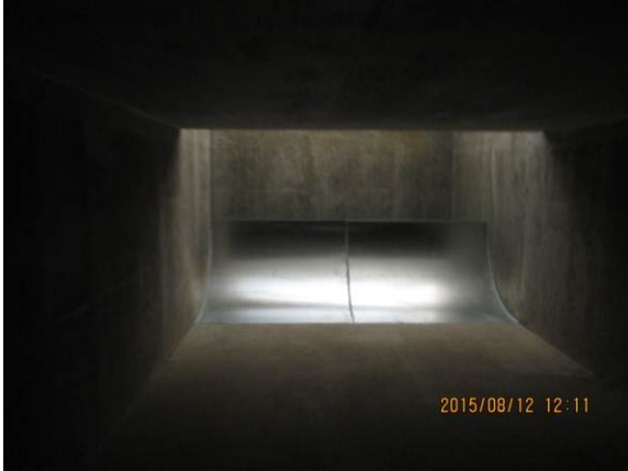
Installation of redesign of ventilation system in progress at Bldg B. LL.
