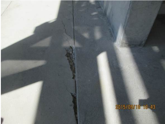
Multiple cracking at joint concrete slab at Parking Garage Level 1.
