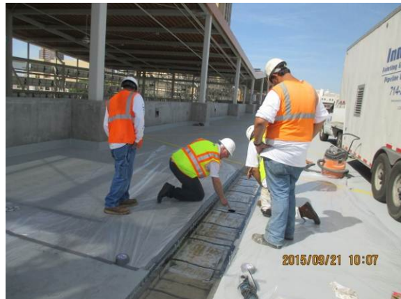
Trench Drain Repair Mock up in progress at Bldg. B Upper Level.
