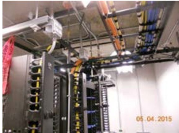
Data Room communication components arrangement at LL Bldg. A.
