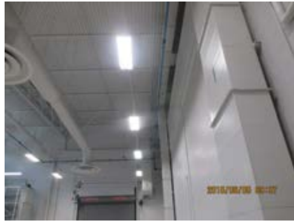
Lighting fixtures powered at Maintenance Building.
