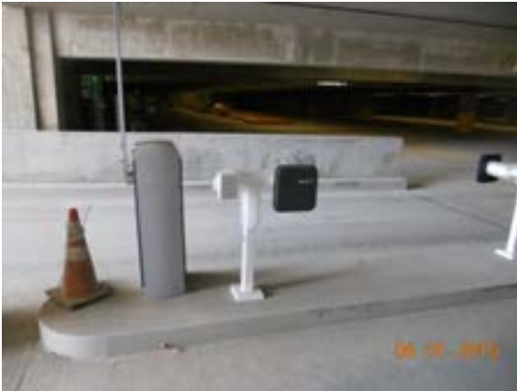
Parking Fare Retrieval System installed at Vignes entrance.
