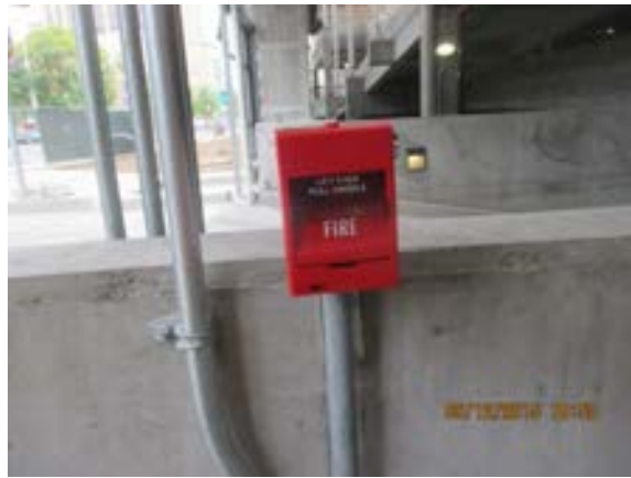
Fire Alarm Device installed at Lyon St Driveway.
