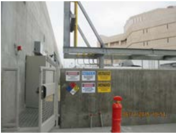
Safety warning signs installed at CNG Facility.
