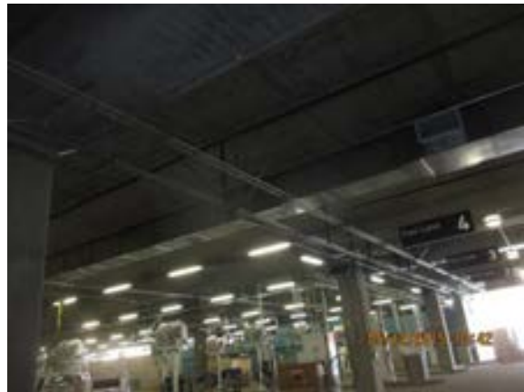
Lighting power operational at Level 1 Maintenance Building.
