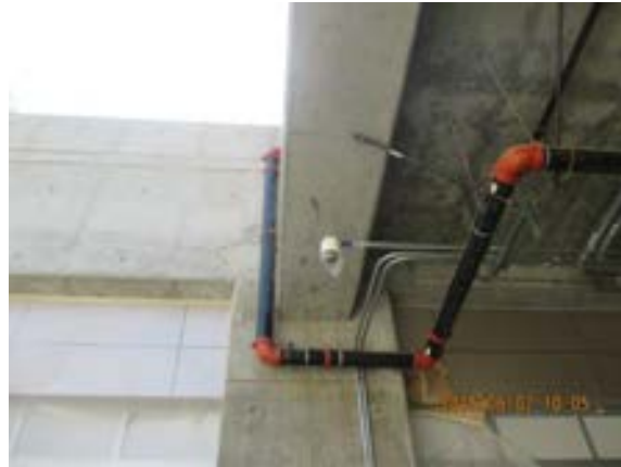
CCTV Camera installed at Maintenance Bldg. under upper level.
