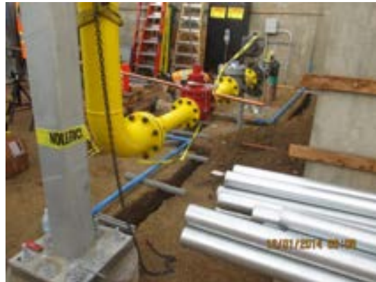
Pressure actuator valves for incoming gas line to CNG Yard.
