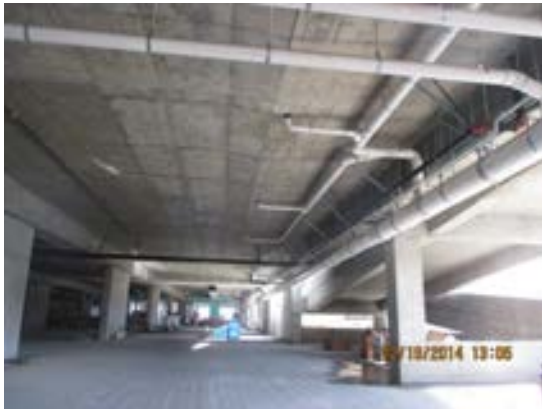
Overhead 18-in storm water pipe at Lower Level Bldg. B.
