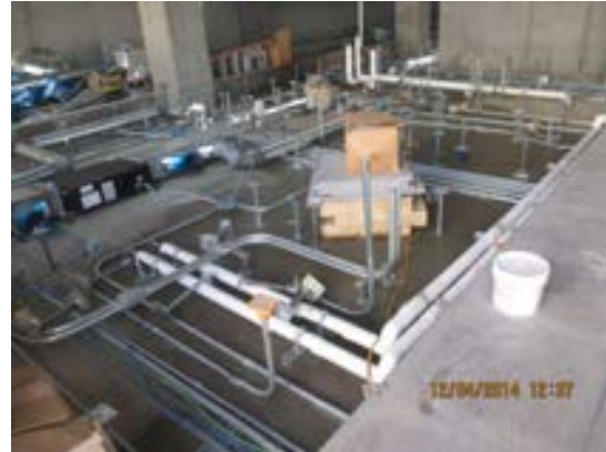
Electrical conduits and water lines under the raised flooring.
