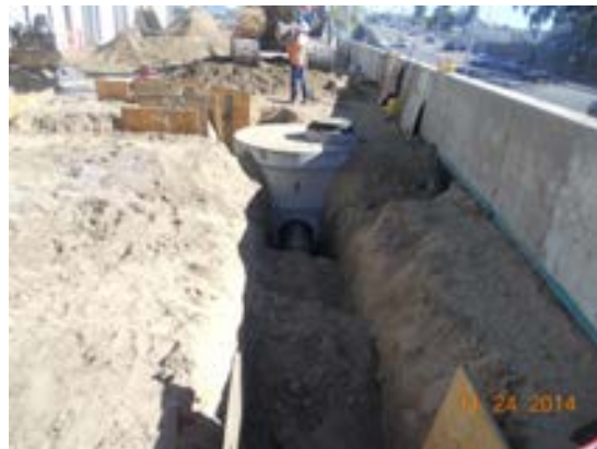
UG water storm line and manholes along Cesar Chavez St.
