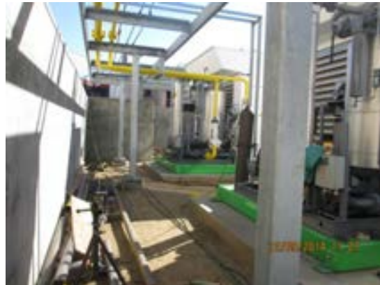
Overhead gas piping and compressors at the CNG Yard.
