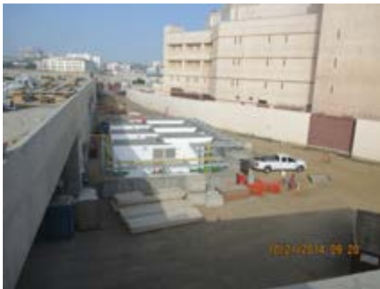
Overhead piping for new dispensers at CNG Yard.
