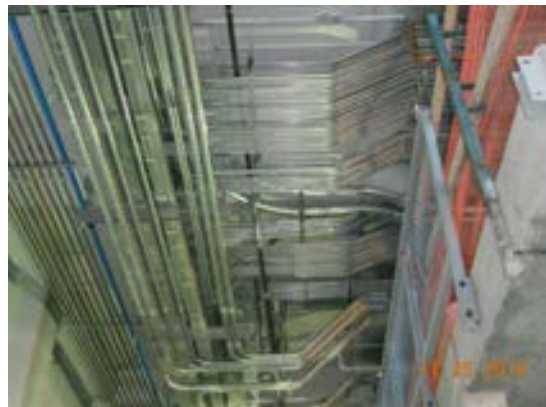
Overhead Elec. Conduits at Level 1 of Parking Garage.
