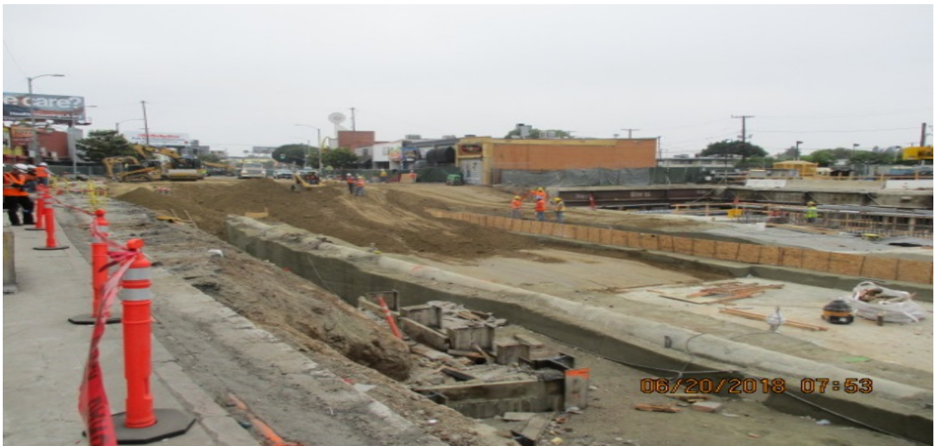
LEIMERT PARK STATION – Backfill and compaction activities at the north end of the station.
