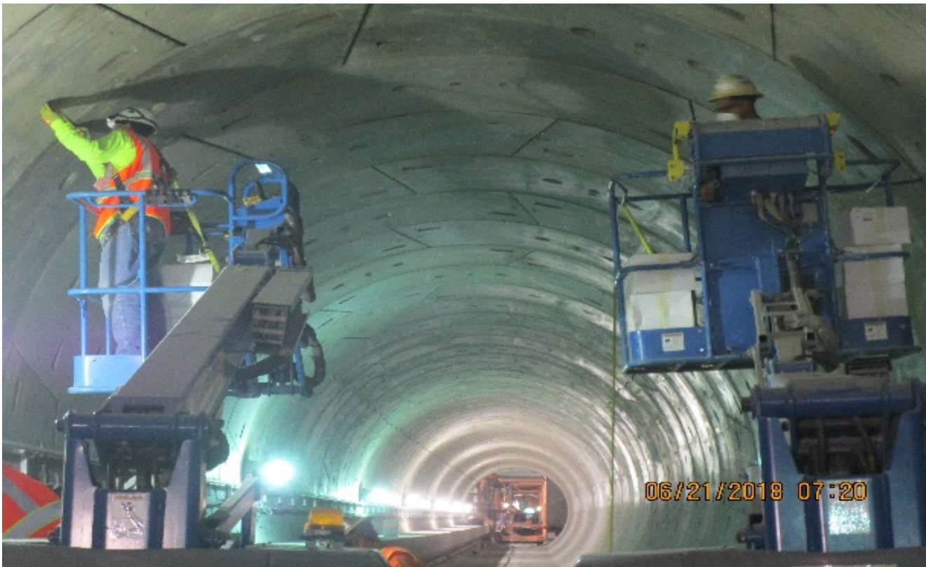
TUNNEL – Installation of the radiating cable brackets in the NB tunnel between Expo and MLK stations.
