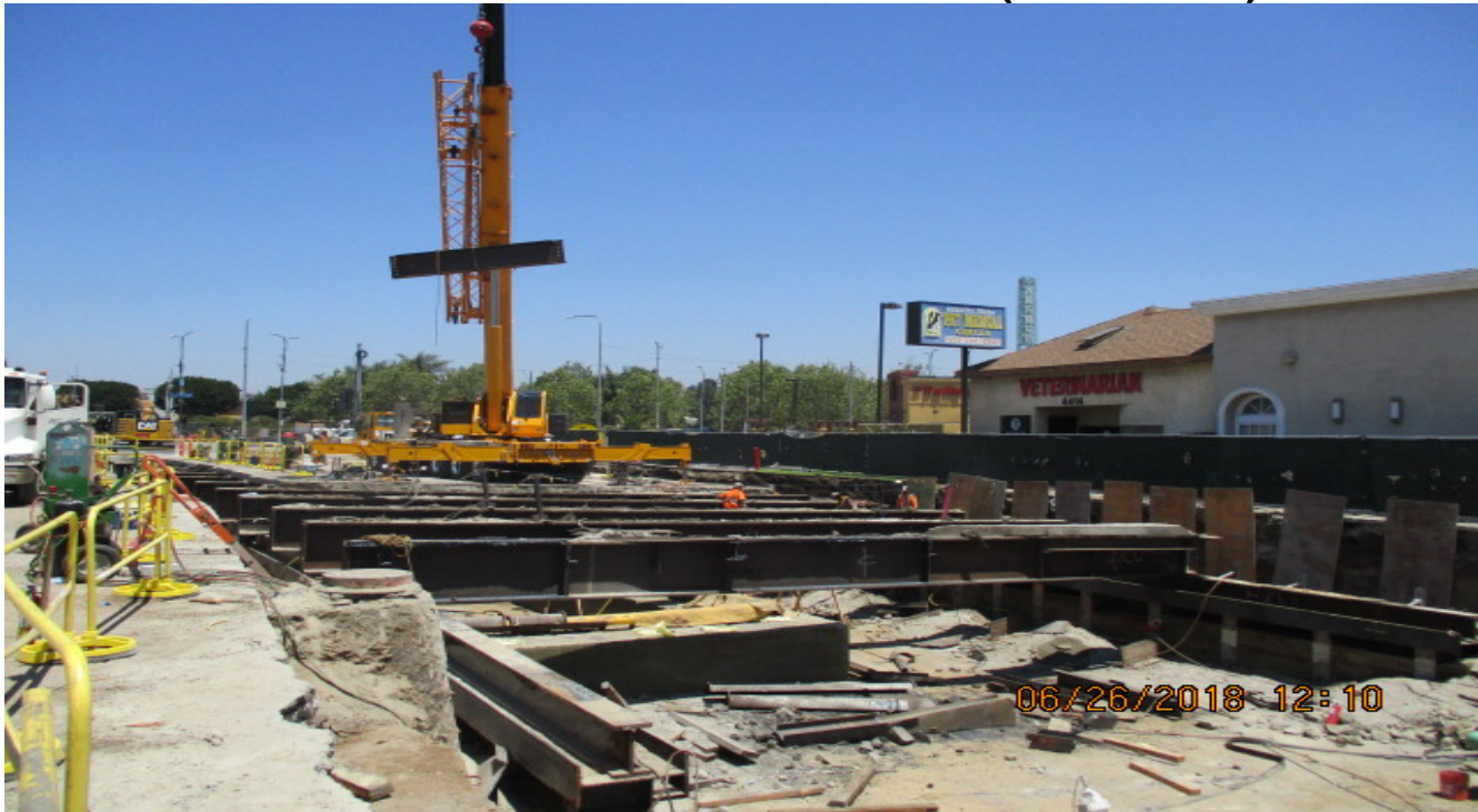
UG4 – Removal of deck beams and panels during the Phase I 43-day closure.
