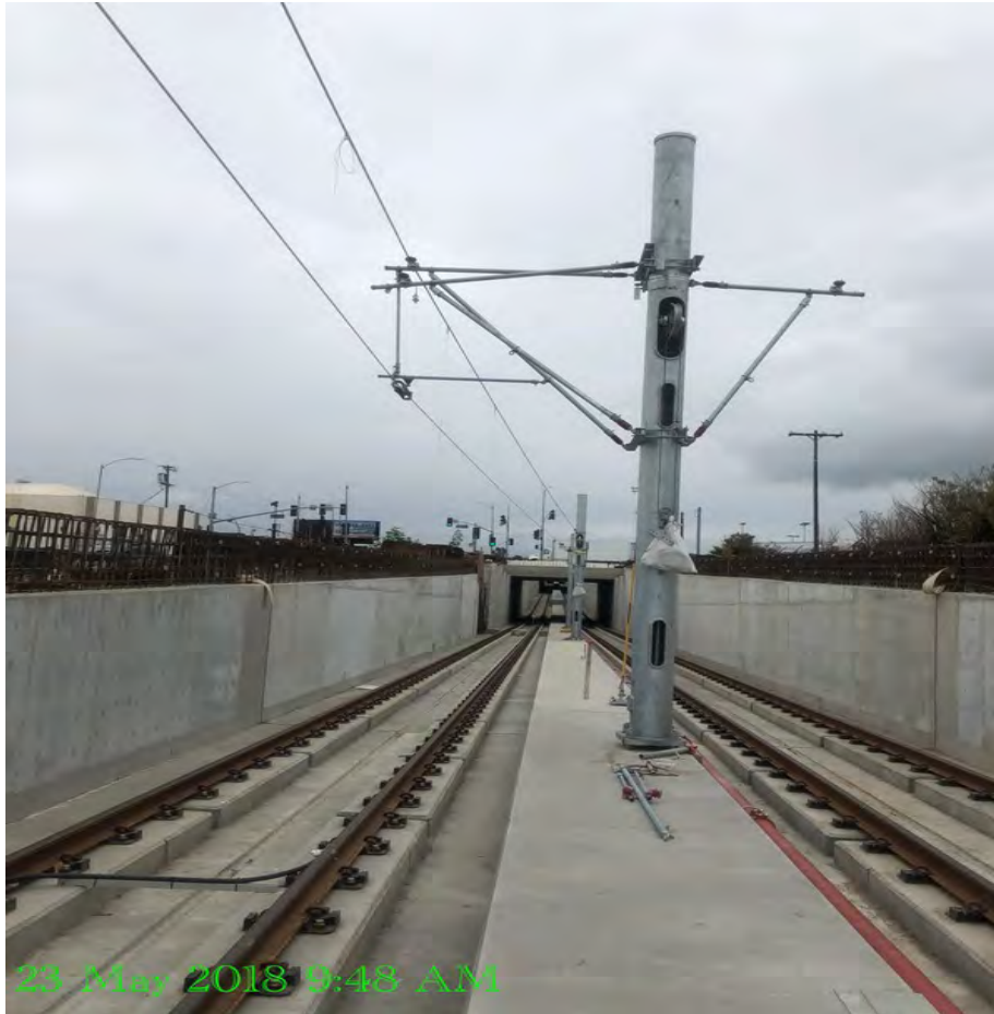
UG1 – track work and overhead catenary system.
