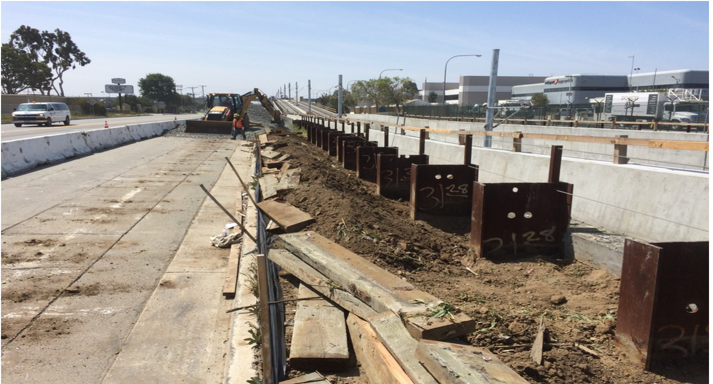
UG1 – Subgrade excavation around the soldier pile beams along the east U-Wall.
