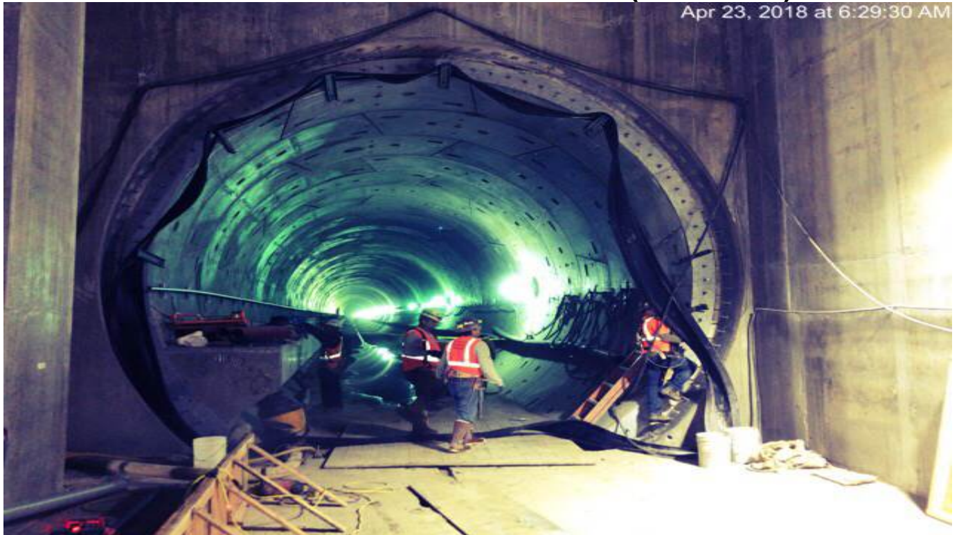
TUNNELING – Installation of omega ring assembly at SB tunnel in Expo station.
