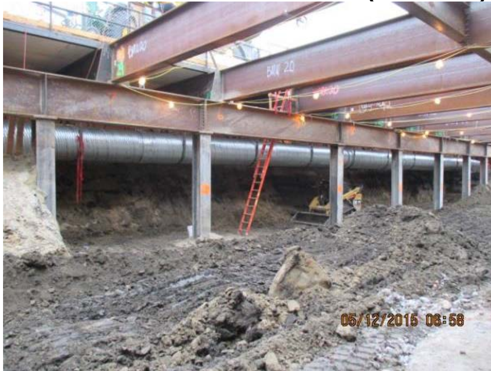
Undermining CMP Storm Drain at MLK.
