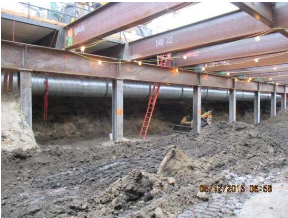
Undermining CMP Storm Drain at MLK.
