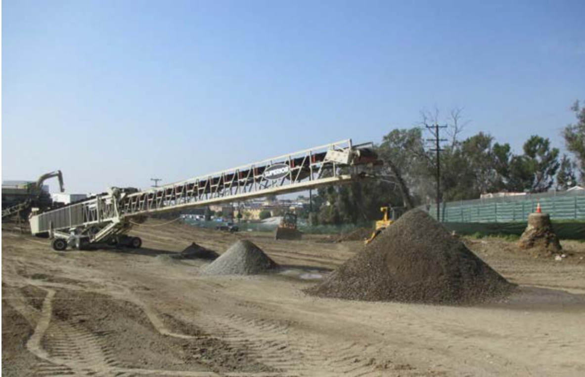
Stock Pile of the Recycled Concrete from the old Century Bridge demolished in July, 2014.
