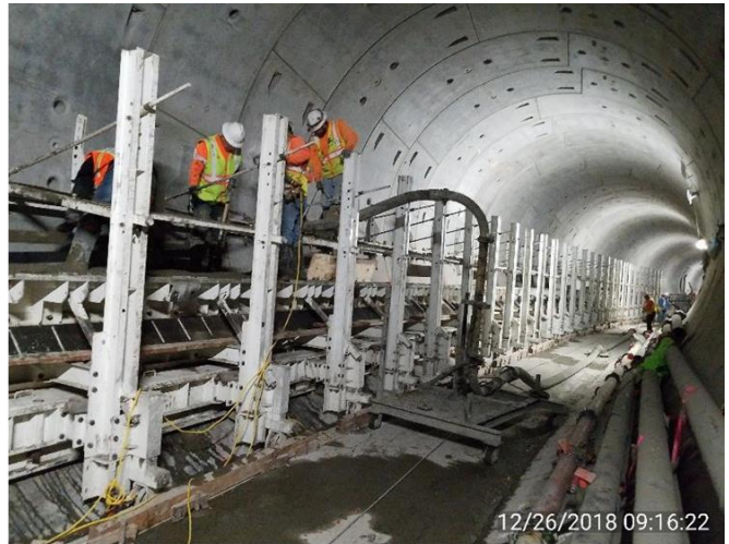
12/26/2018 09:16:22 Left Tunnel walkway concrete placement from future Little Tokyo/Arts District Station towards Historic Broadway Station
