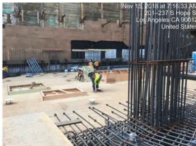
Layout of embeds at concourse level deck at Grand Av Arts/Bunker Hill Station
