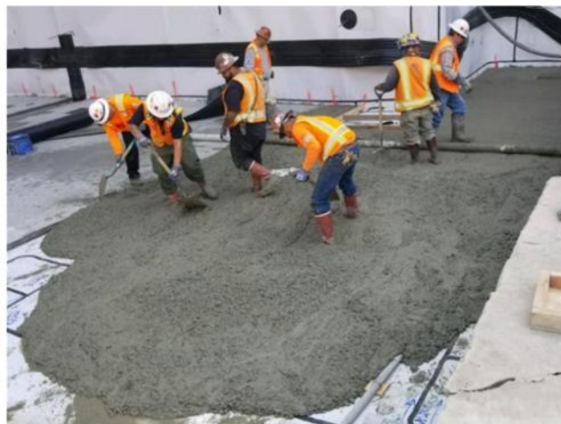
Protection slab placement at ancillary level of future Little Tokyo/Arts District Station
