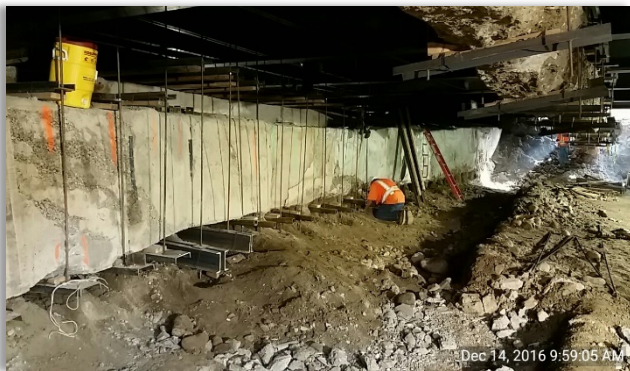
Utility hanging under 2nd Street decking
