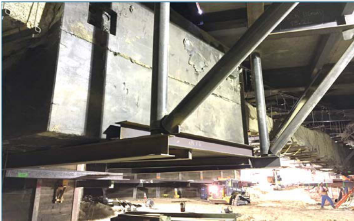
Hanging Utilities under Wye
