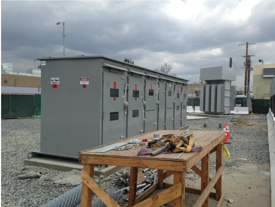
C0980 Contract – Substation at Mangrove Yard
