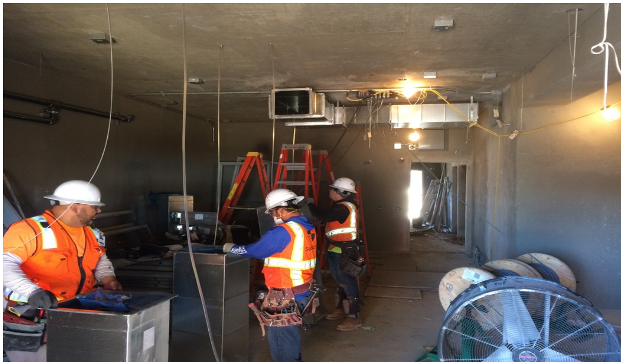
AVIATION/CENTURY STATION – Installation of the HVAC ducts inside the Service Building TC&C room.
