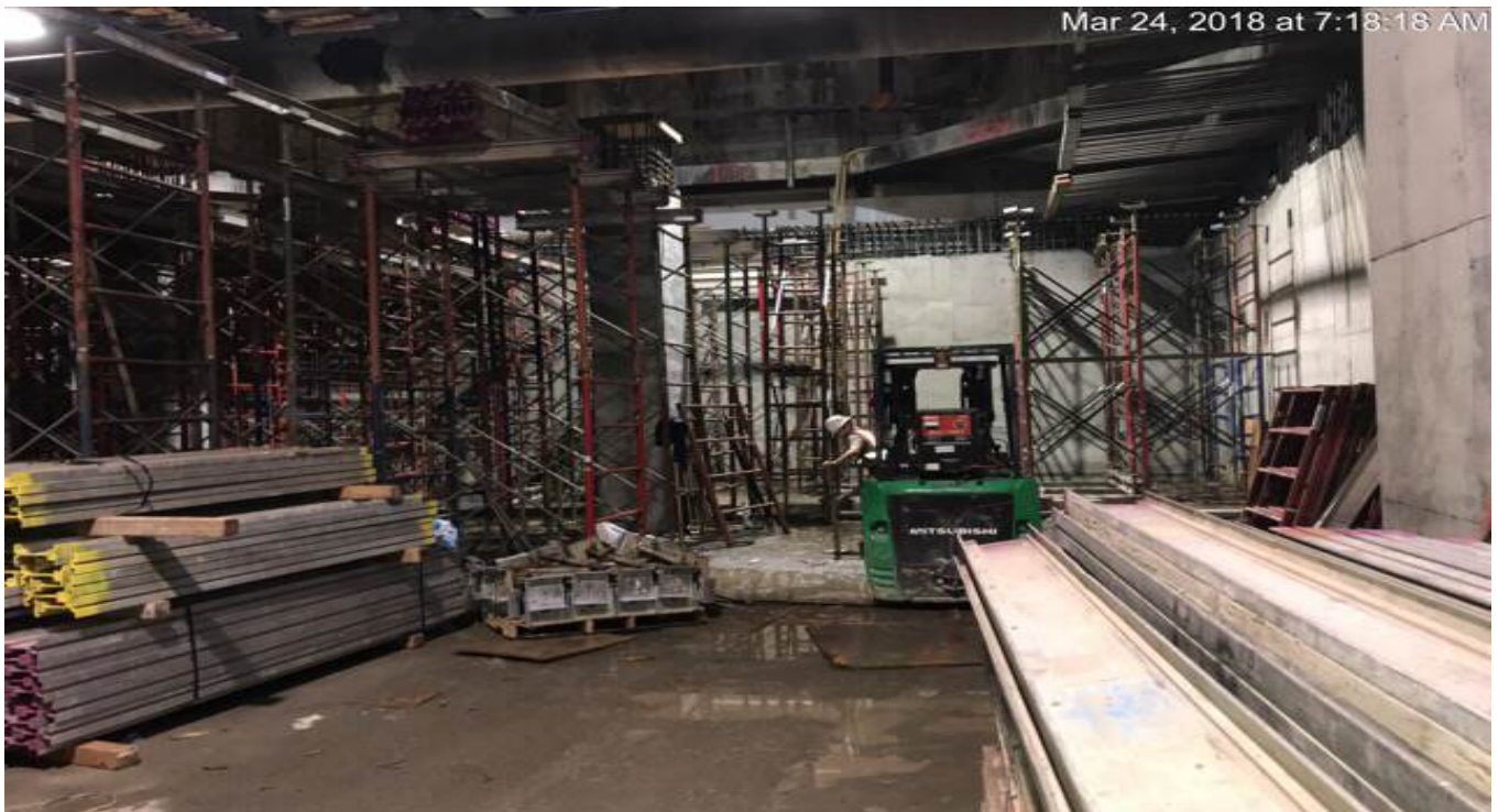
MARTIN LUTHER KING JR. STATION Installation of false work for phase 2 roof construction.
