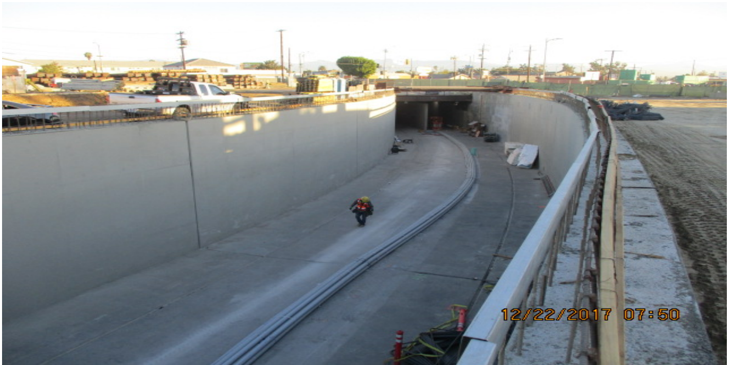
UG#3 - Previously installed walkway conduit at the south portal.
