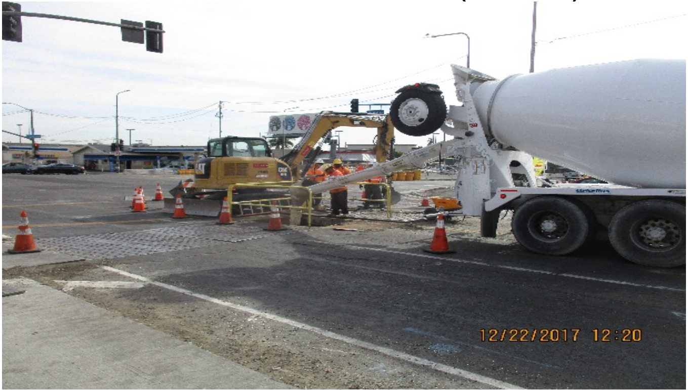
PARK MESA - Placement of storm drain invert at manhole #16 at Slauson Ave HYDE.
