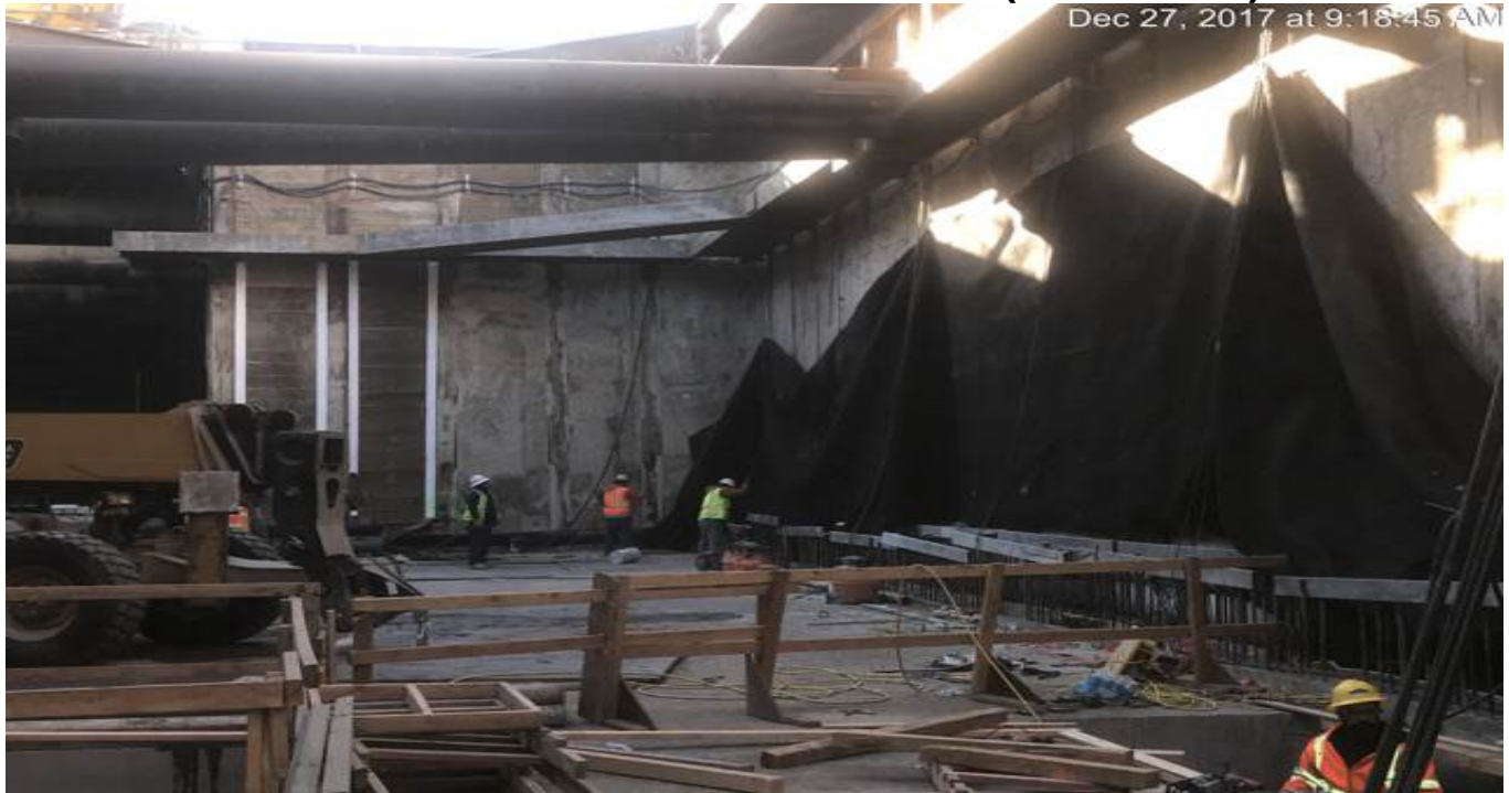
MARTIN LUTHER KING JR. STATION – Installing waterproofing along the west concourse level walls.
