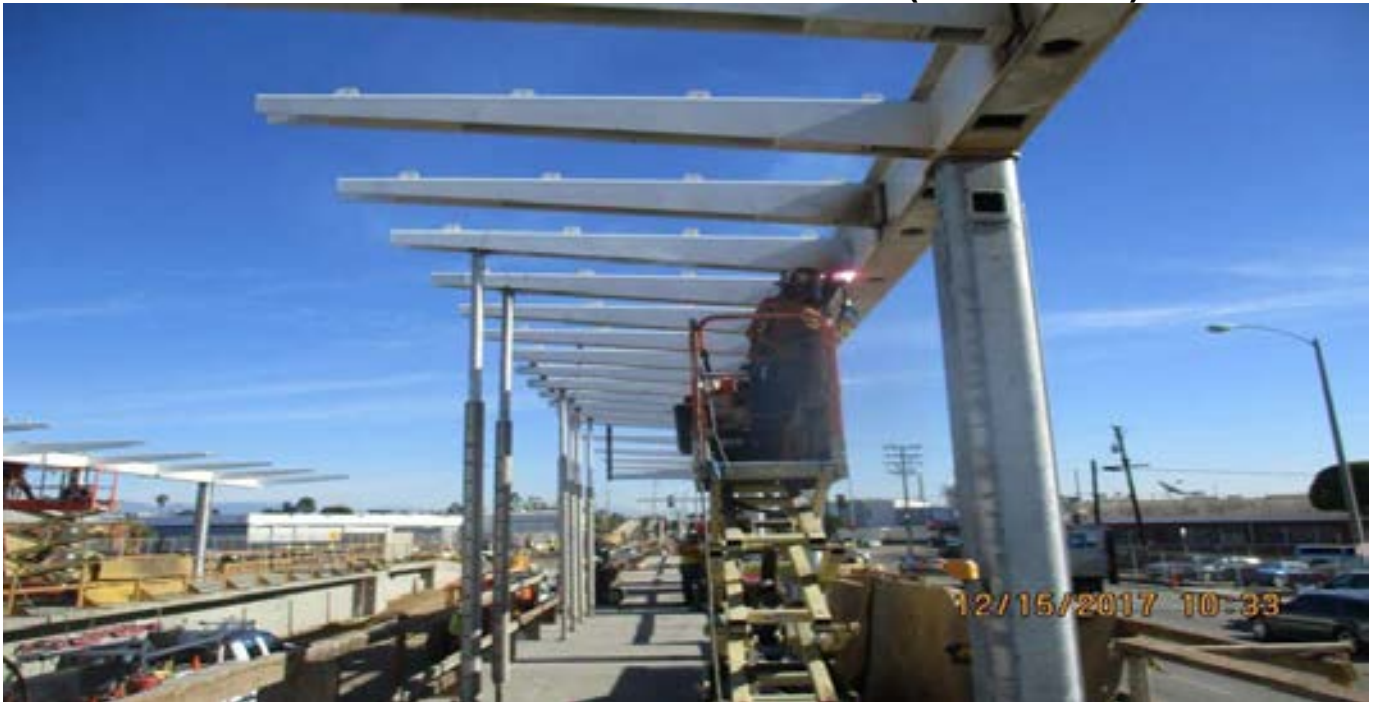
WESTCHESTER STATION – Crew continued splice welding of canopy frames and column to canopy girder FP.
