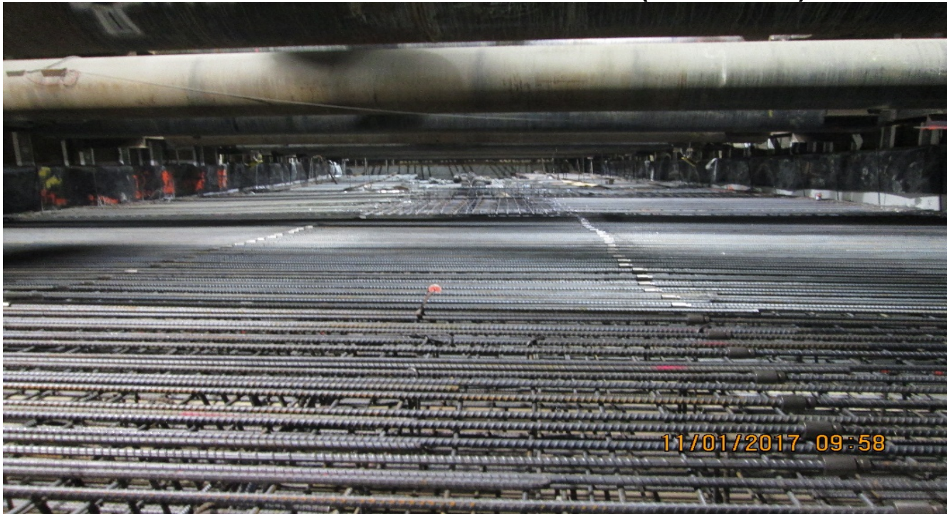
UG4 – Installing rebar for roof sections R-28 thru R-25, south of Vernon portal.
