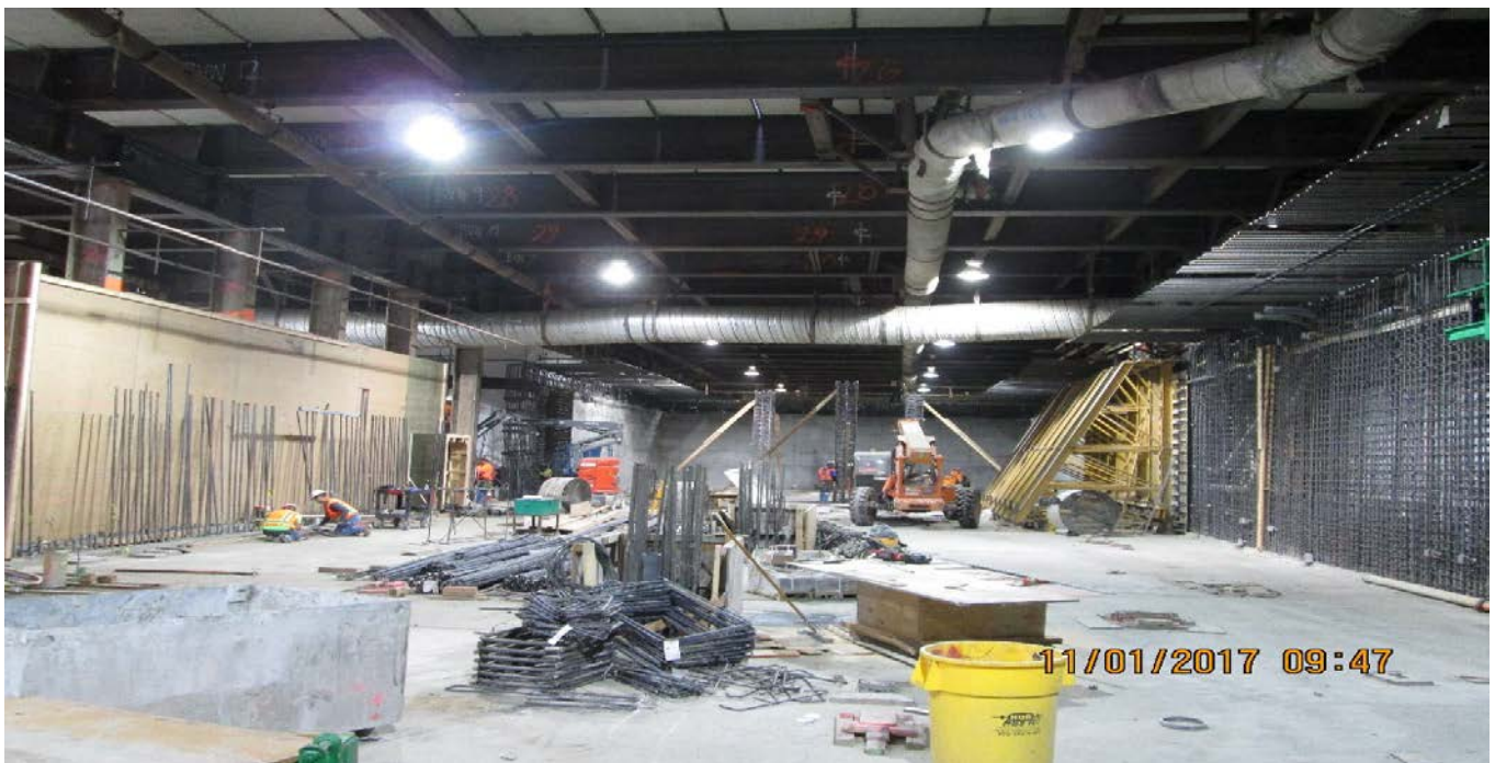
LEIMERT PARK STATION - Installing formwork and rebar along south concourse level walls.
