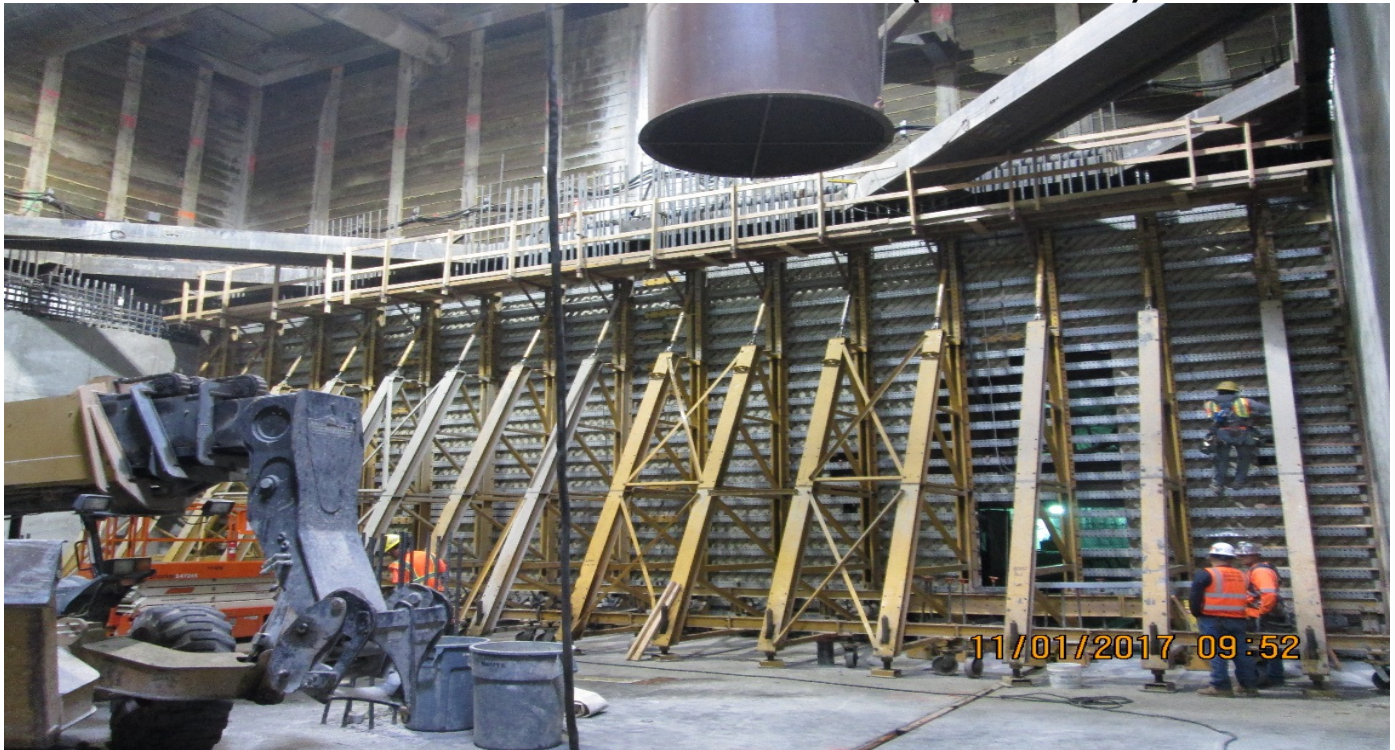
LEIMERT PARK STATION – Installing rebar for lower walls in the north hammerhead.
