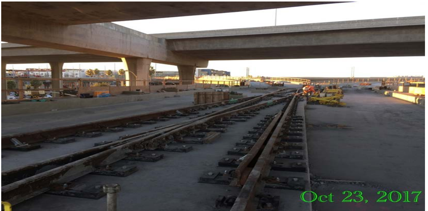
GREENLINE UNDERPASS – Crew installing slobber plate, rail fasteners and rail restraining rail at movable switches.
