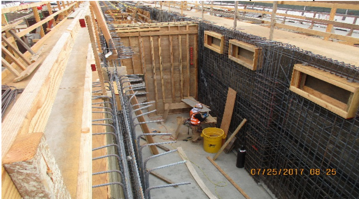
HYDE PARK STATION- Installation of formwork for walls at TC&C room. _PARK MESA- Placement of asphalt south of Slauson Ave.
