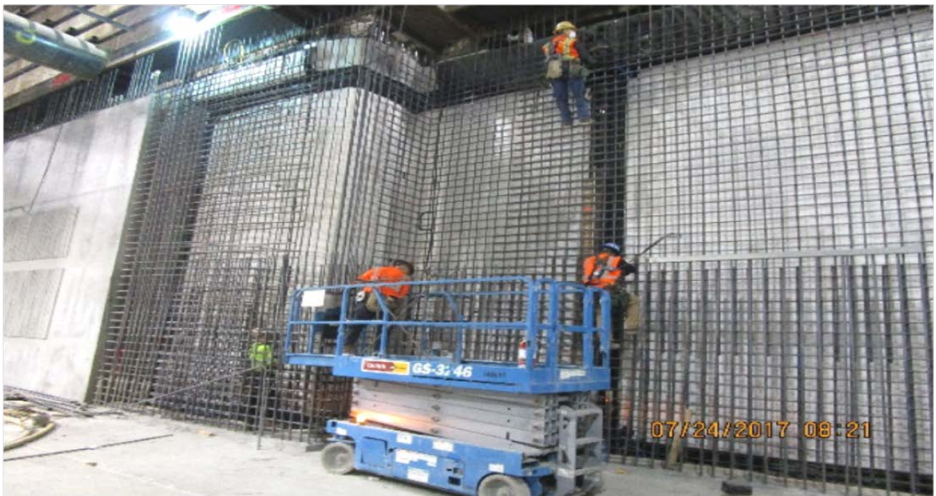
MARTIN LUTHER KING JR. STATION – Installation of formwork and rebar for invert level walls.
