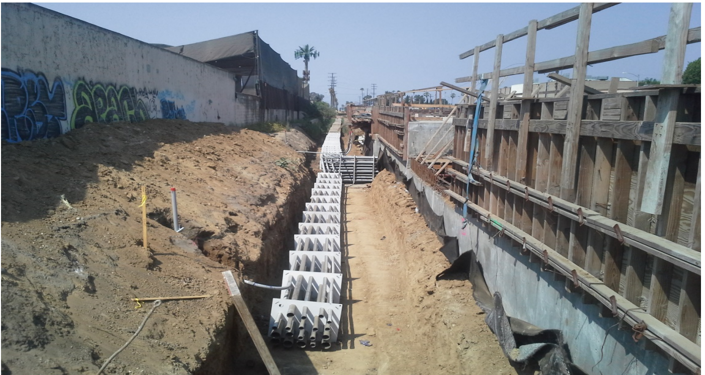
WEST STATION - HDPE installation and backfill adjacent to the west platform walls complete. Crews installed the mainline ductbank along the eastern perimeter of the center platform.
