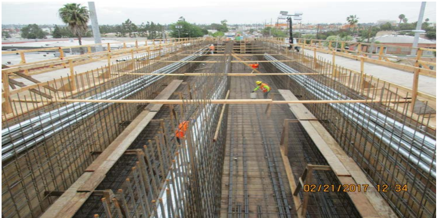
(AG-5) I-405 BRIDGE -Integrity rebar placers continued installing superstructure reinforcement and continued installing post tensioning ducts. Crews began installing girder stem formwork.
