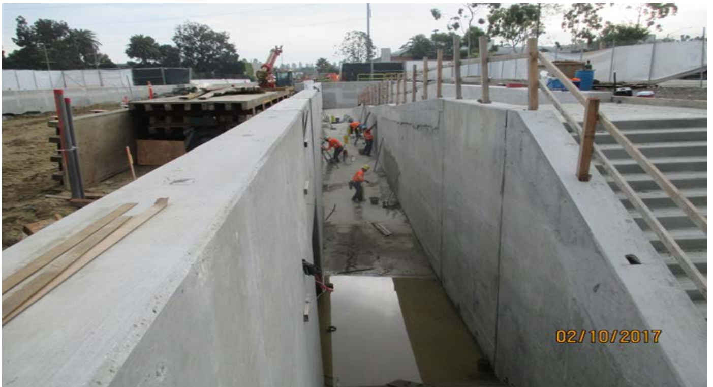
(AG-7) FCBC Pedestrian underpass - Finish work ongoing. South Access Ramp and Stairs.
