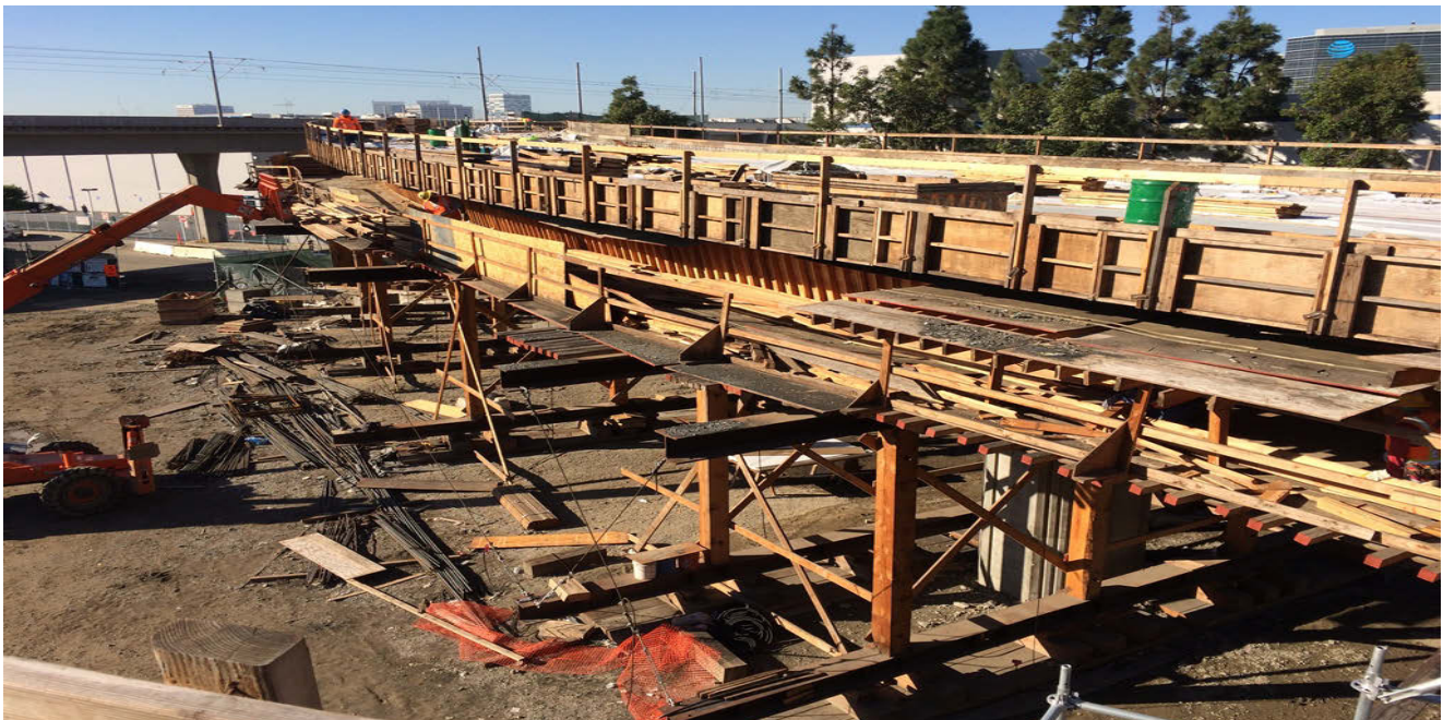
GREENLINE UNDERPASS – Frame A: overhang formwork removed and PT tendons installed by DSI.
