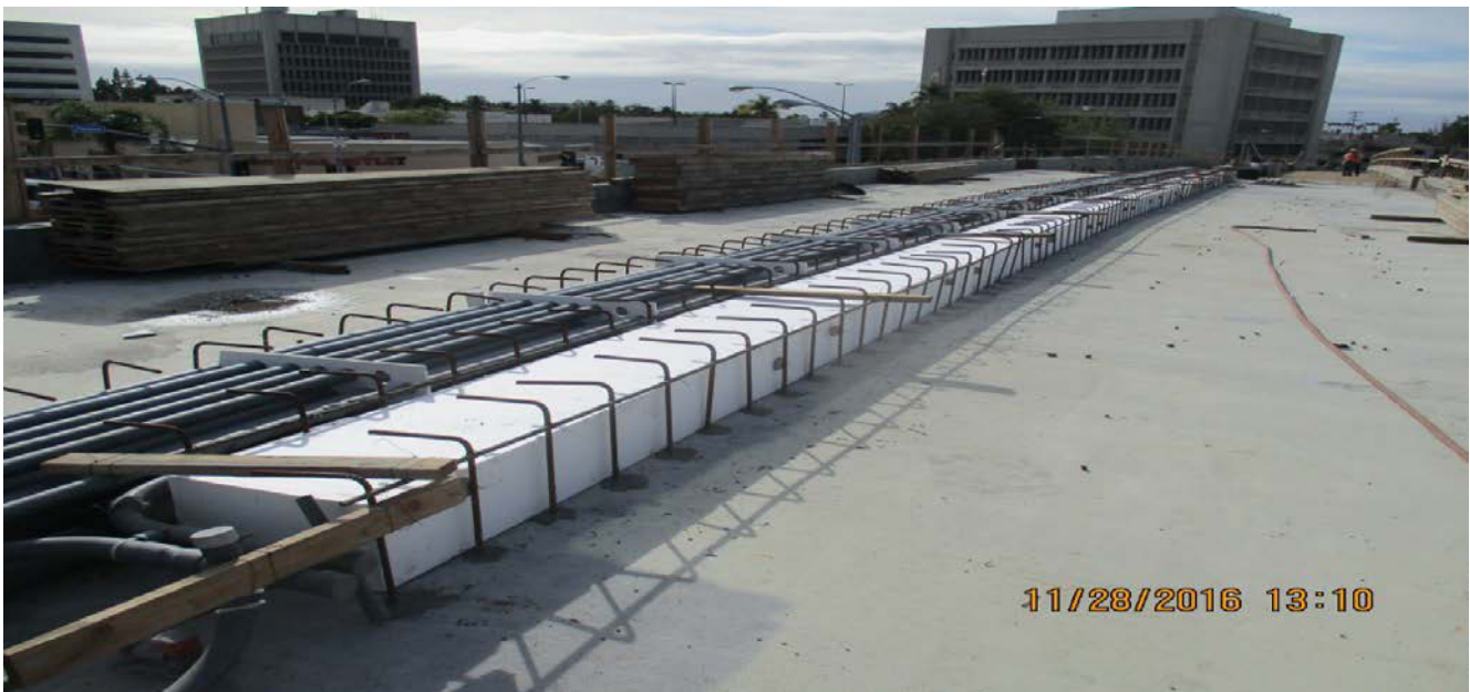
(AG-6) LA BREA BRIDGE – Crews continued to drill and bond the Emergency walkway/ CS ductbank.
