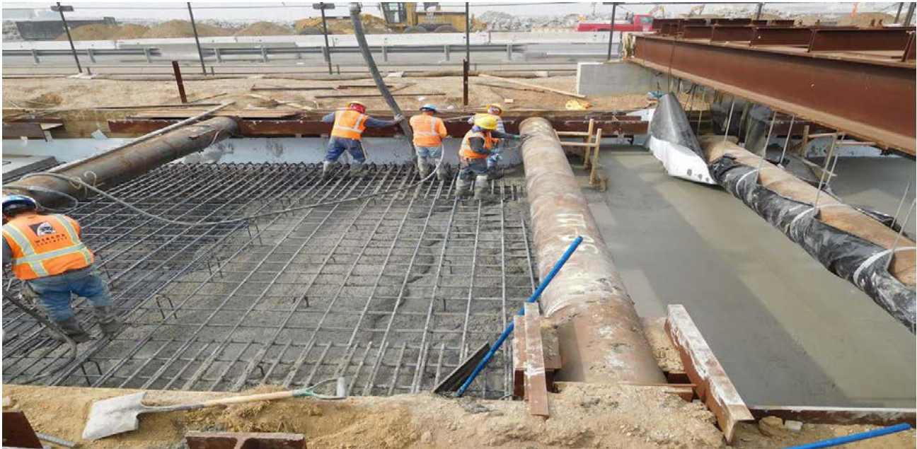
UG#1 – Crews continue with sequential construction at Underground Guideway 1 progressing from south to north.
