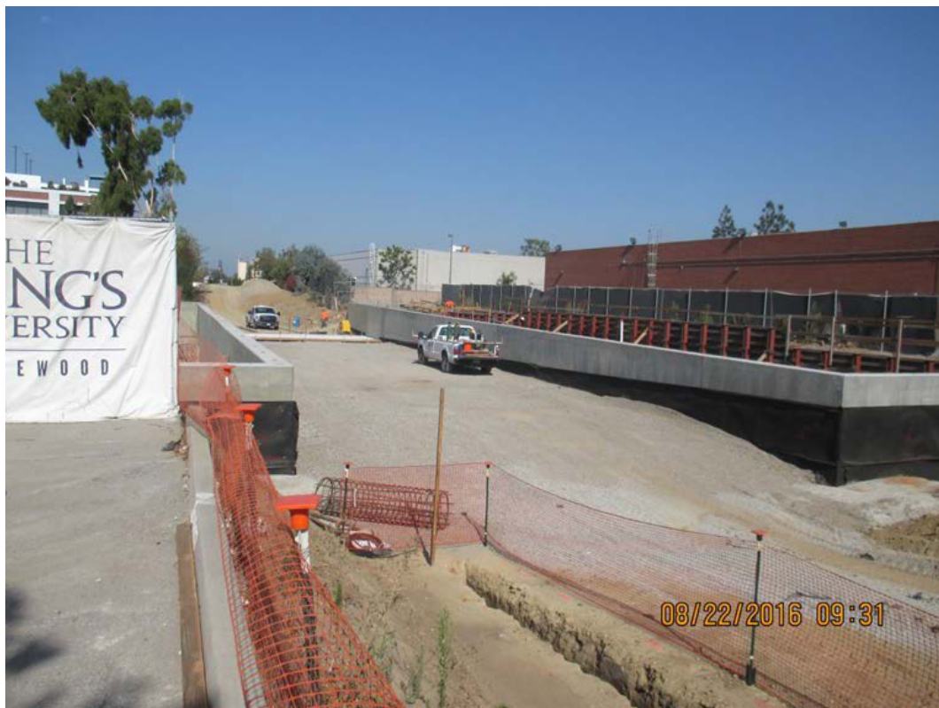
FAITHFUL CENTRAL BIBLE CHURCH PEDESTRIAN UNDERPASS – Backfilling and compaction testing between exterior ramps.
