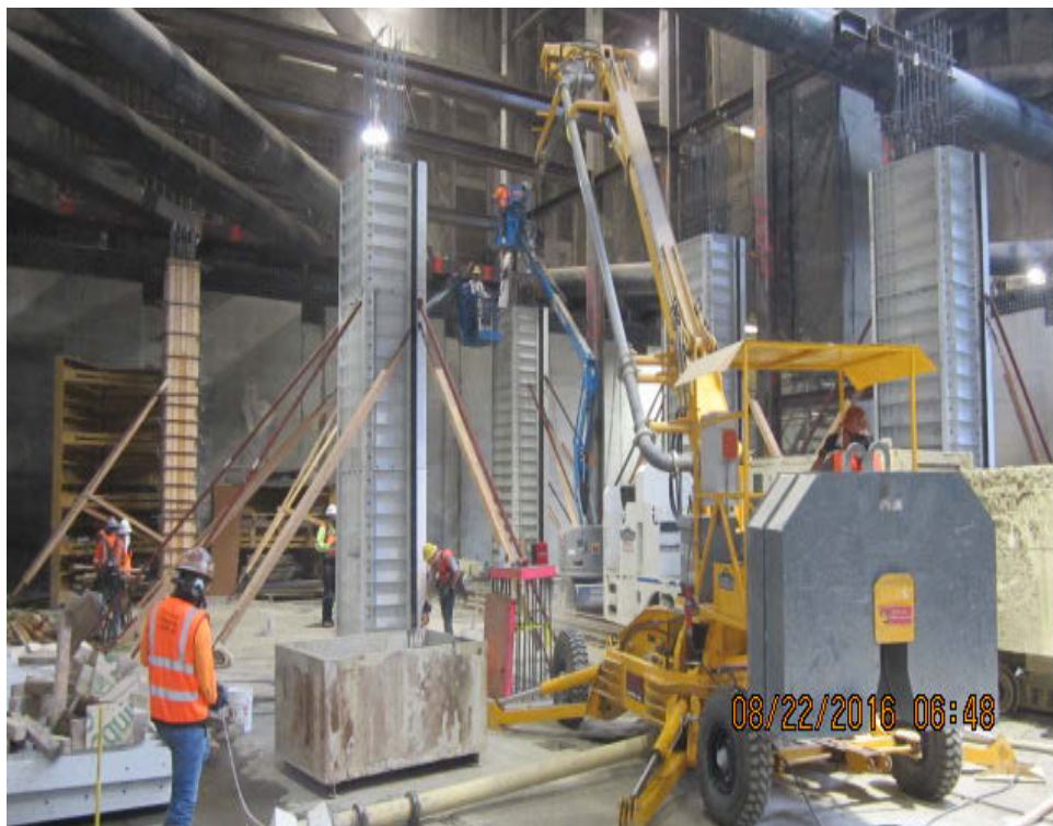
EXPOSITION/CRENSHAW STATION – Placement of lower invert columns at the north end of station box.
