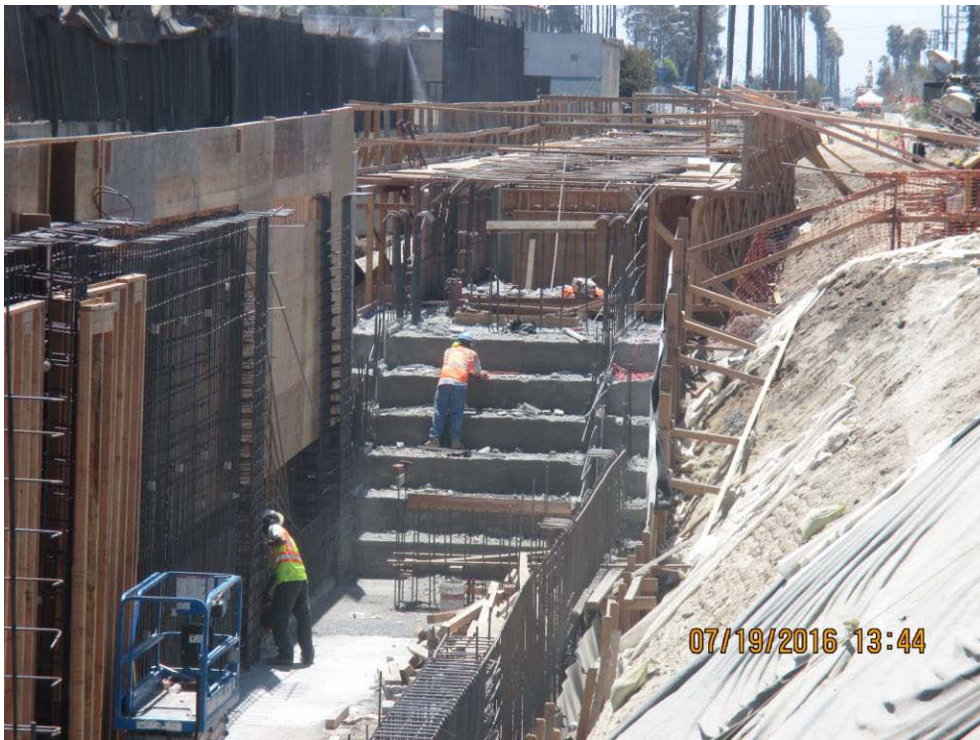
FAIRVIEW HEIGHTS STATION - Crews continued installing rebar and formwork for Southern retaining wall for the subterranean TC&C room.
