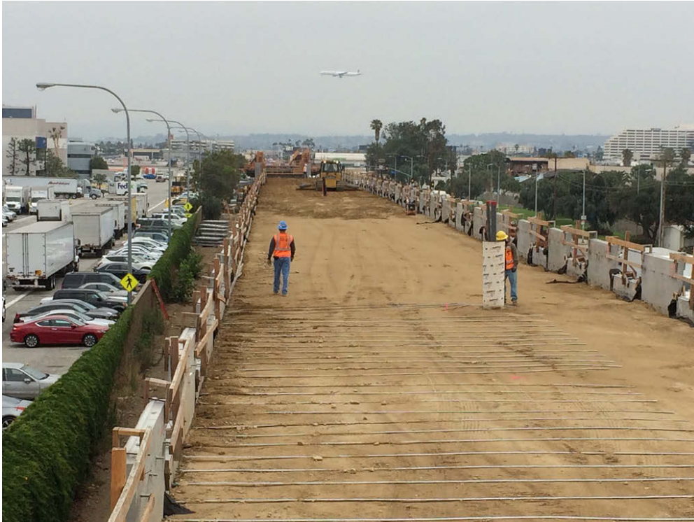
MSE Wall 17L&R (North of Imperial Highway): Crews worked on galvanized strap placement, embankment backfill and compaction.
