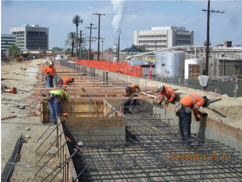
DOWNTOWN INGLEWOOD STATION - Crews worked on installing formwork and rebar for the station's footing and grade beams.
