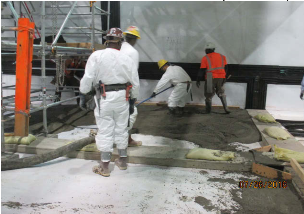
LEIMERT PARK STATION - Placement of protection slab at east side of station box.
