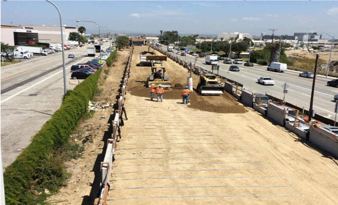
MSE WALL 17L&R (North of Imperial Highway): Subgrade preparation, leveling pad placement, precast panel erection, galvanized strap placement, embankment backfill and compaction testing ongoing.
