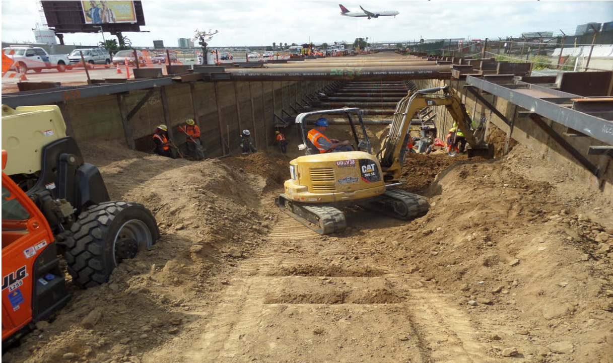
UNDERGROUND GUIDEWAY 1 – Excavation bracing and lagging installation continues at the north end.
