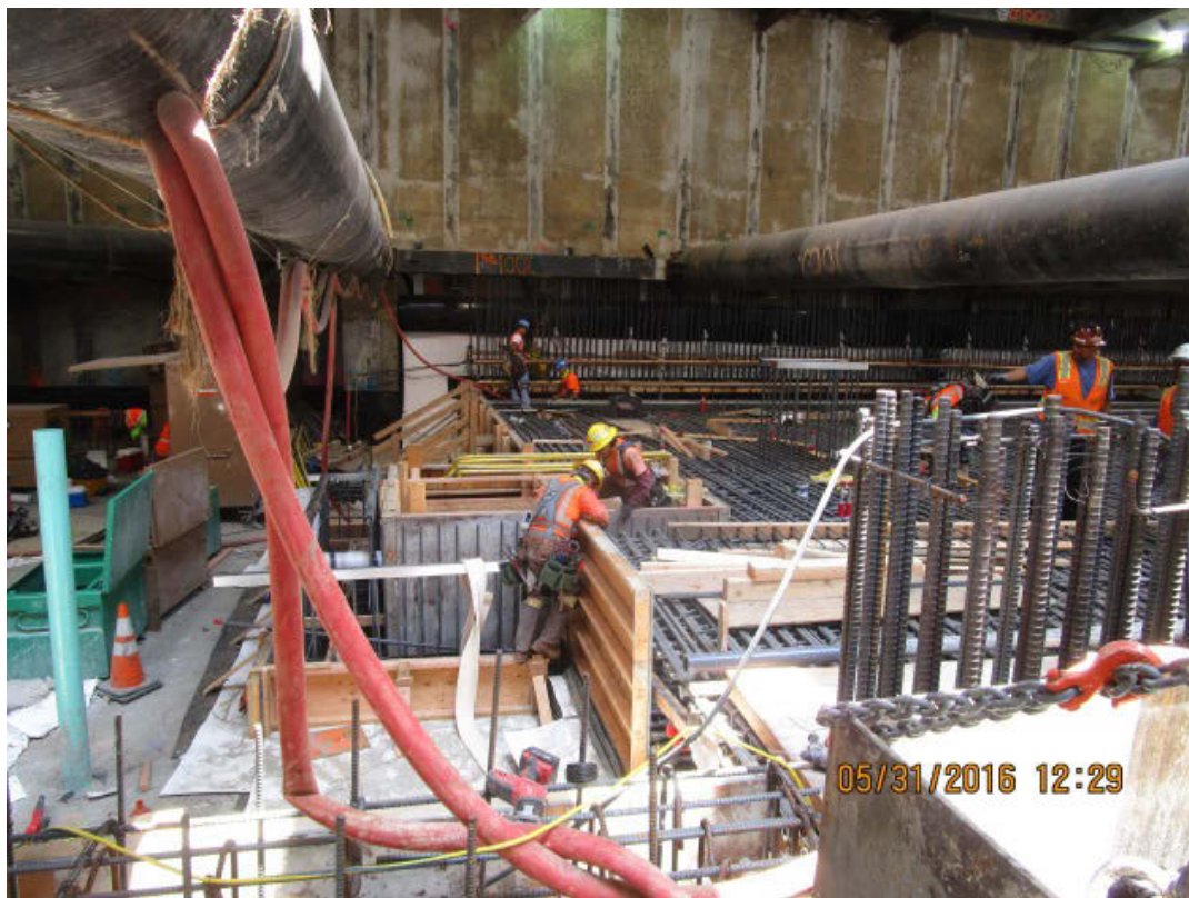
MARTIN LUTHER KING JR. STATION – Installation of electrical conduits, plumbing, and rebar at north end of station.
