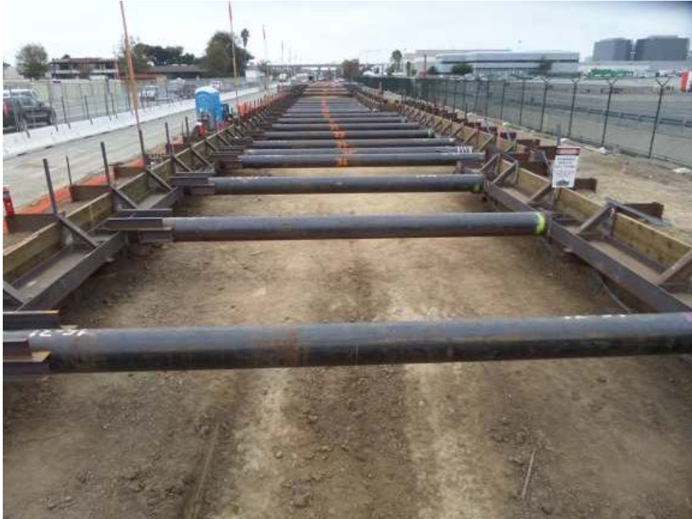
UG#1 - Struts and wales being installed per plan. Excavation continues down to tier 2
