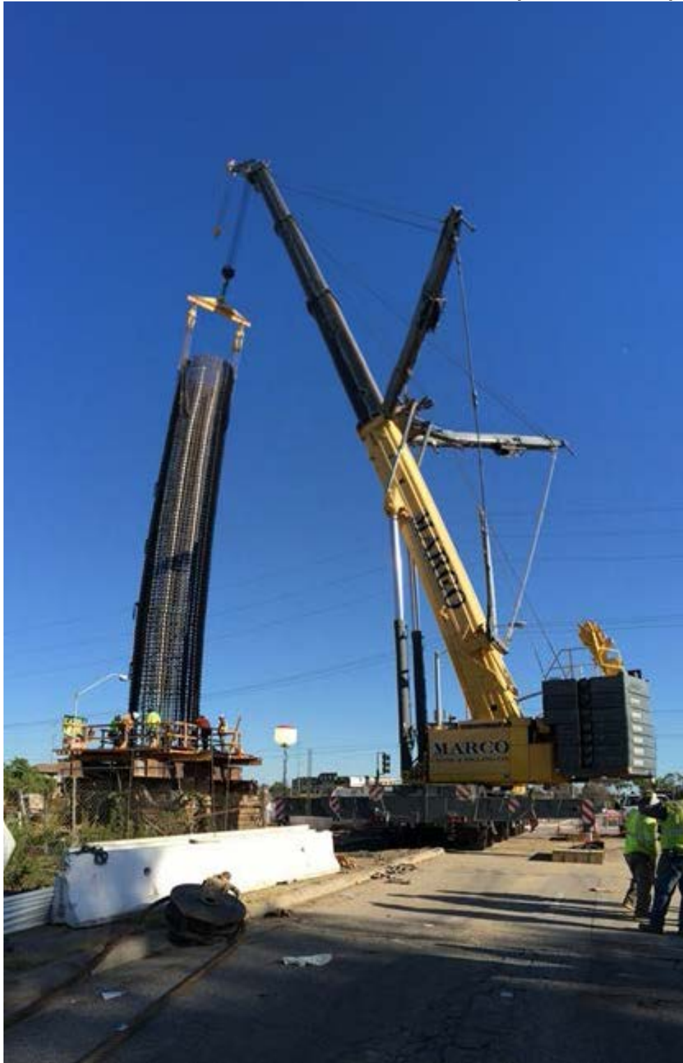
I-405 Bent 2 CIDH cage was set. Column cage being installed 09/24/15, followed by the concrete pour on 09/26/15.
