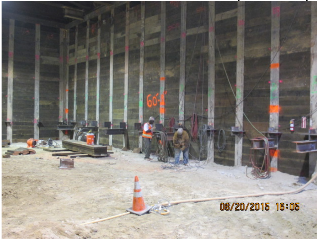
LEIMERT PARK STATION – Installation of T-packs and look outs for Tier 1 support.
