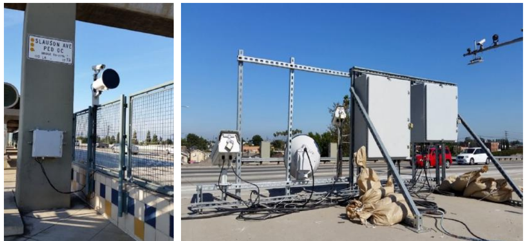
Figure 18: VPDS Camera and Equipment
