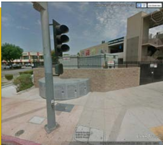
Figure 2-7. Typical TPSS Facility
