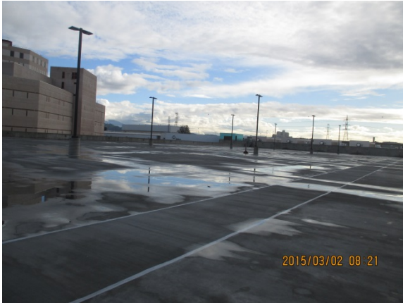
Rain pounding residue at Parking Garage Upper Level.
