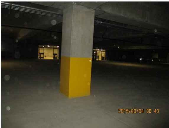
Power now activated in Parking Garage Lower Level.
