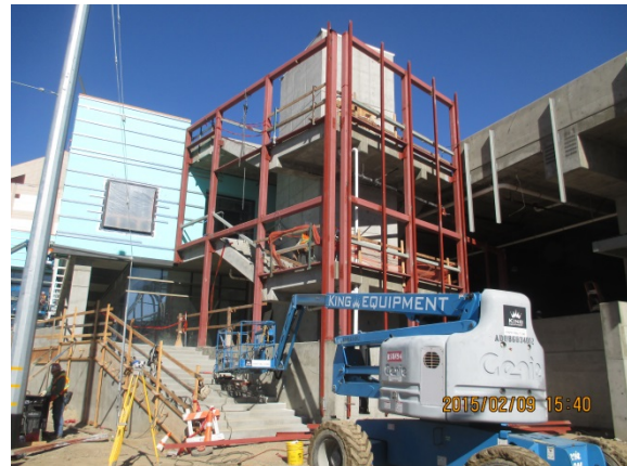
Stairs #1 Concrete Phase Done. Red Structural Steel. Installation in Progress at South of Transp. Bldg.
