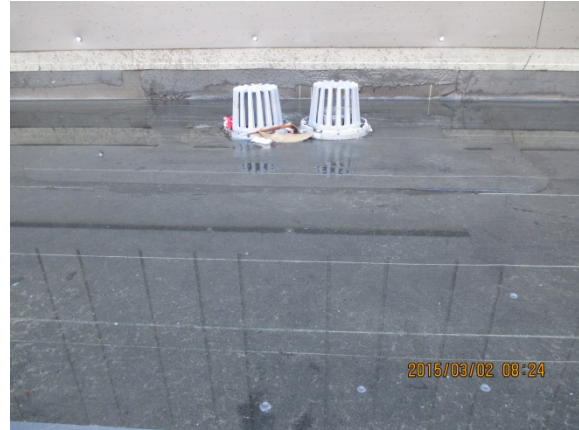
Roof Drain clogged by rain at Vegetated Area.
