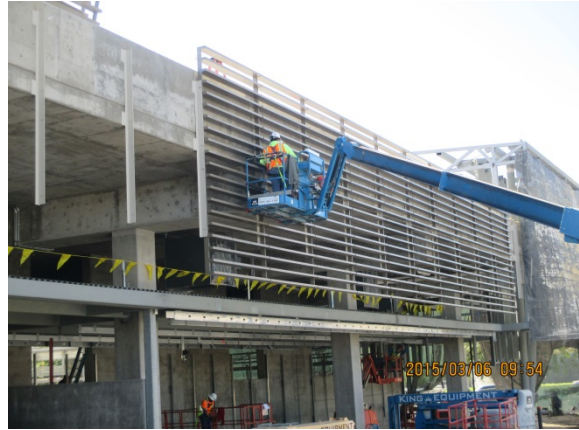
Installation of horizontal steel membranes at exterior west side of Parking Building.
