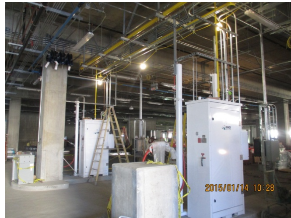
Overhead CNG gas piping at Fuel Island in Parking Garage.
