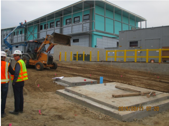
Jelly Fish Tank and Water Reservoir in place at Utility Yrd Area.
