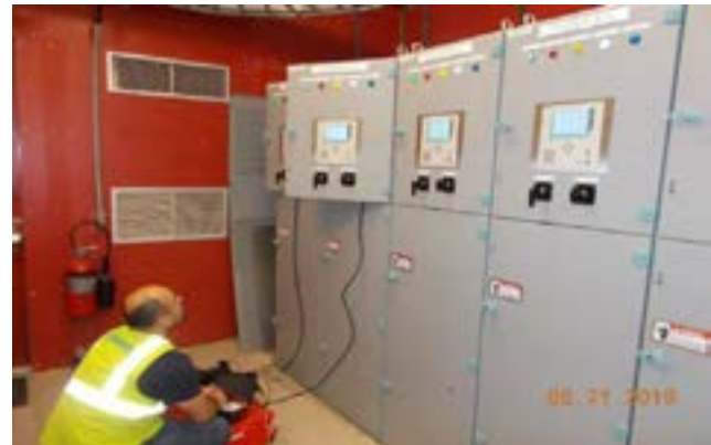
TRACTION POWER SUBSTATION #1 – Performing transfer trip test.
