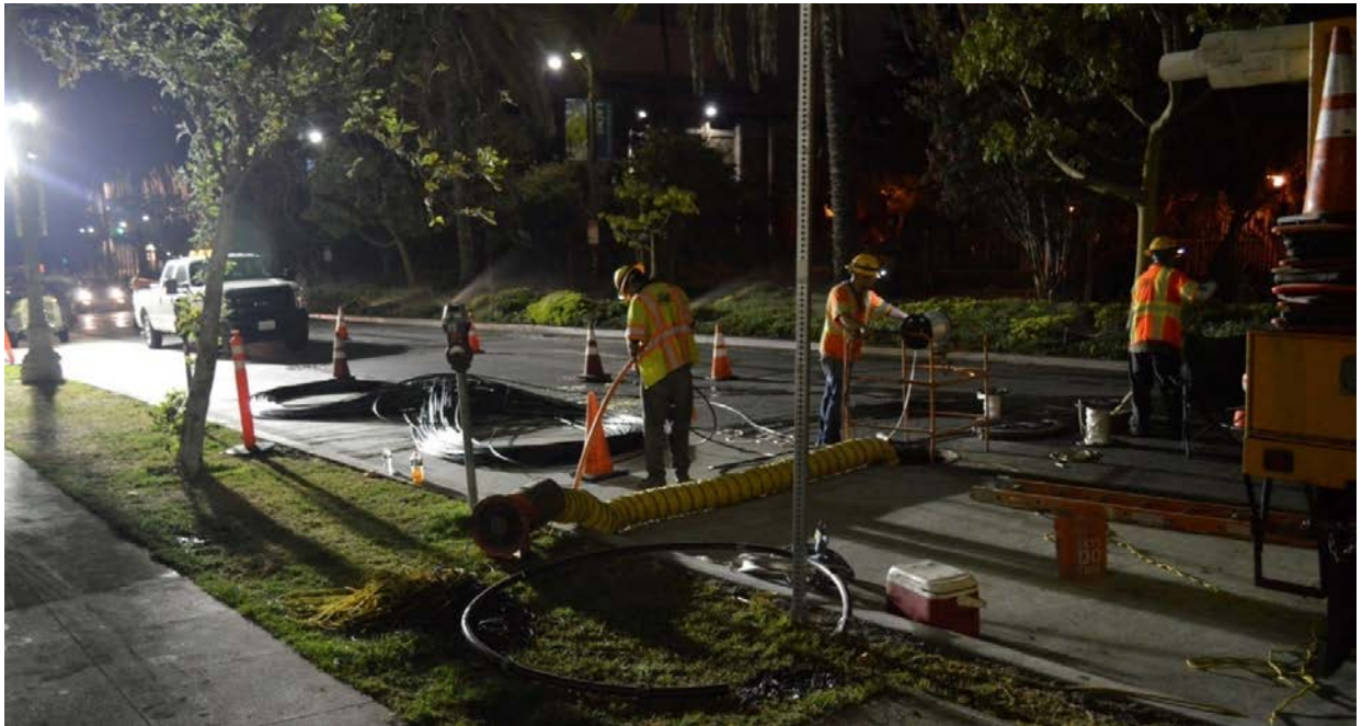
CES Performing Fiber Optic Work on Wilshire Boulevard in the City of Beverly Hills
