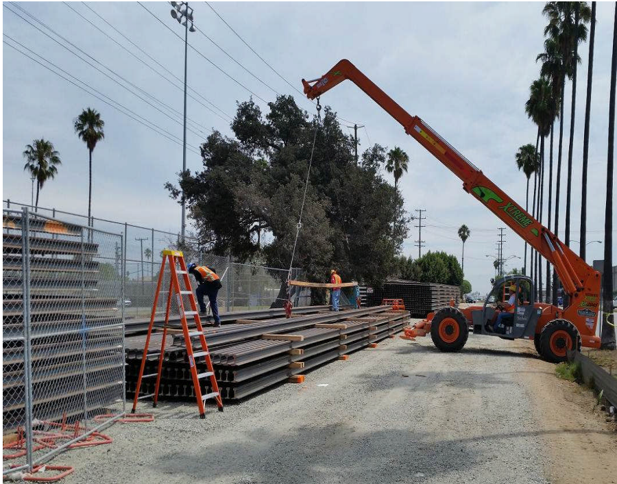
Segment B (Crenshaw/Vernon Station to Hindry Station) – Rail delivery and stock pile at the Florence laydown yard.
