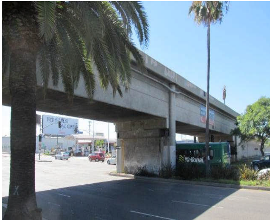
Defunct railroad bridge on Century Blvd and Aviation prior to the demolition.
