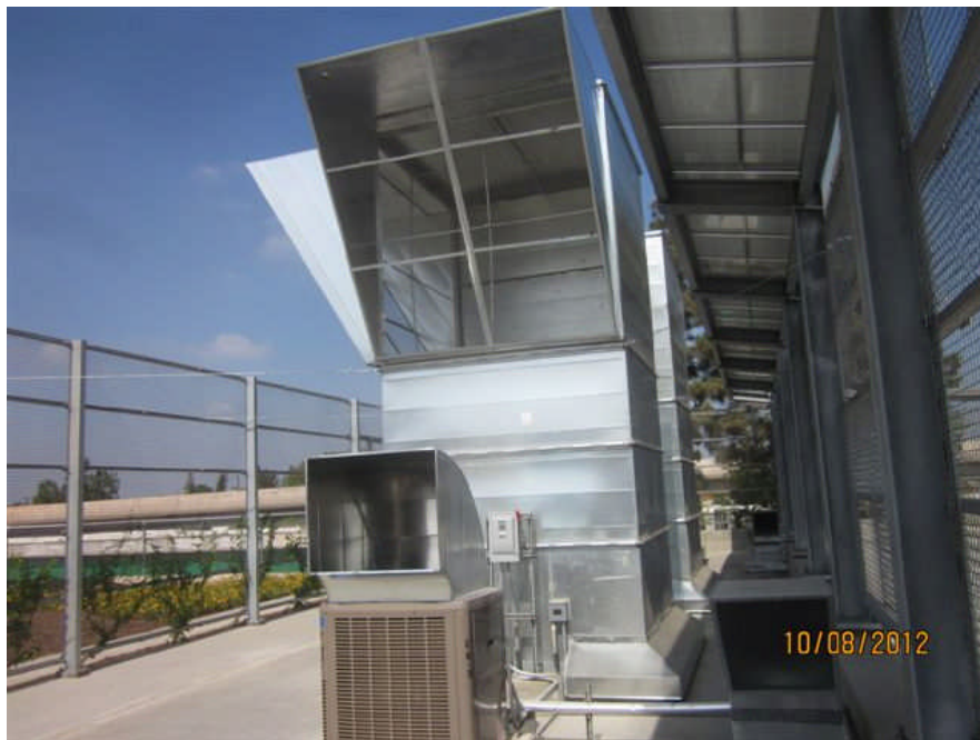
Guy cables on exhaust fans stacks.
